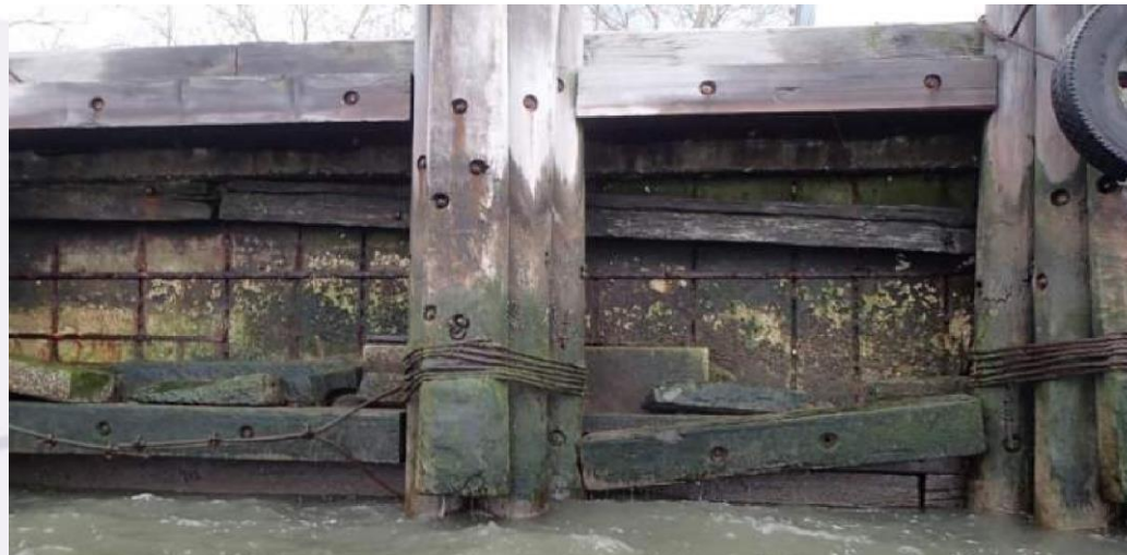
LOSS OF GRANITE BLOCK FASCIA
