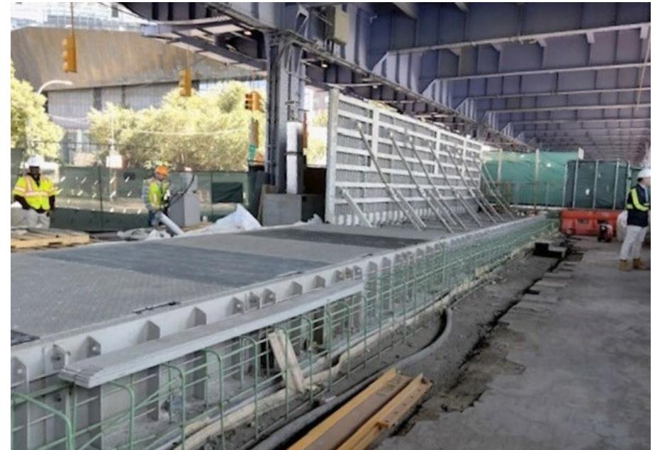
Flip up gate in partially deployed position – September 2024
