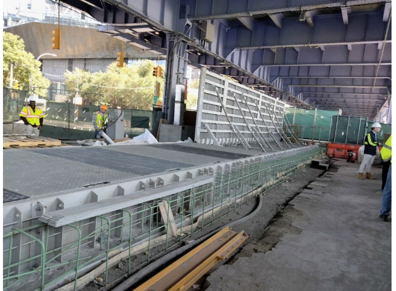
Flip up gate in partially-deployed position – September 2024
