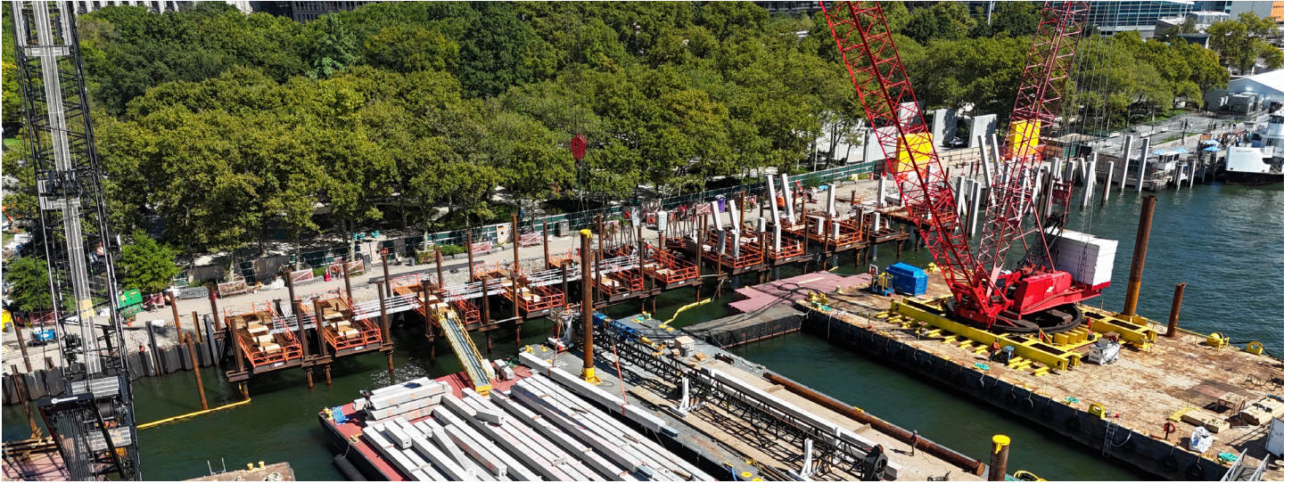
Image: Aerial view of precast concrete pile installation setup and material staging on barges.
