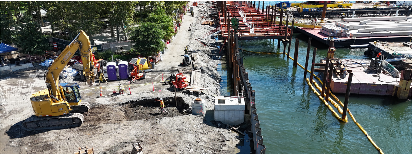
Image: Aerial view of upland drainage structures and storm water retention improvements adjacent to future wharf structure.
