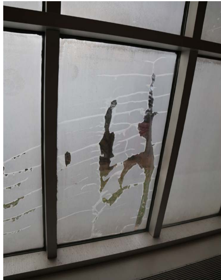
Interior detail of with deteriorating plastic film
