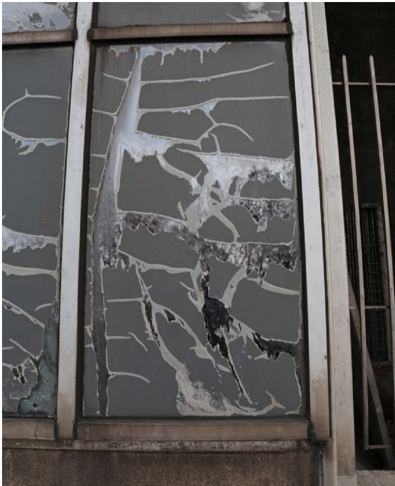
Exterior detail: deteriorating plastic film and corroding curtain wall framing
