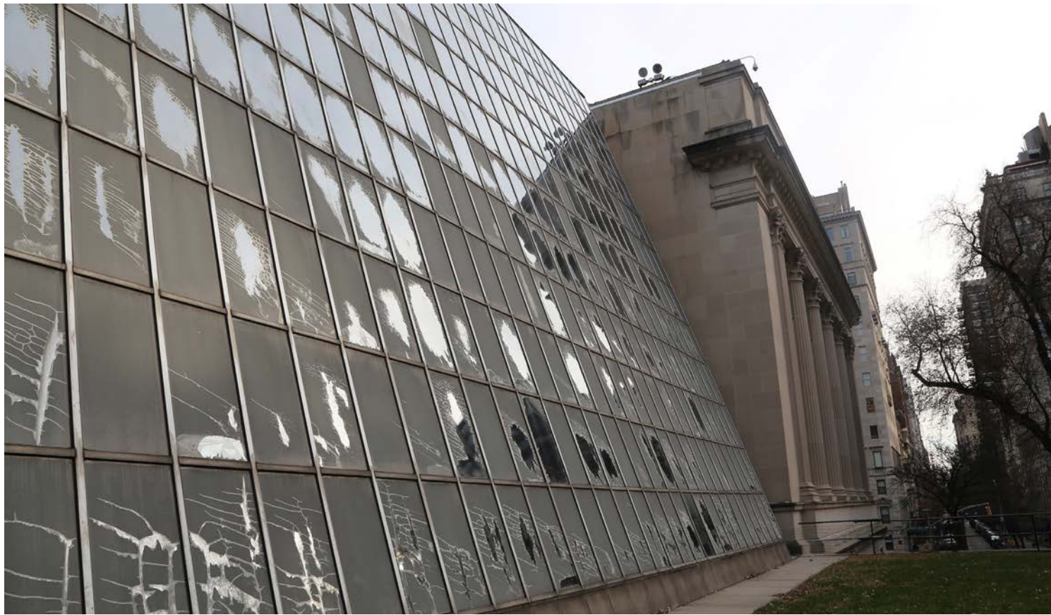
Existing condition: exterior with deteriorating tinted plastic film on glass
