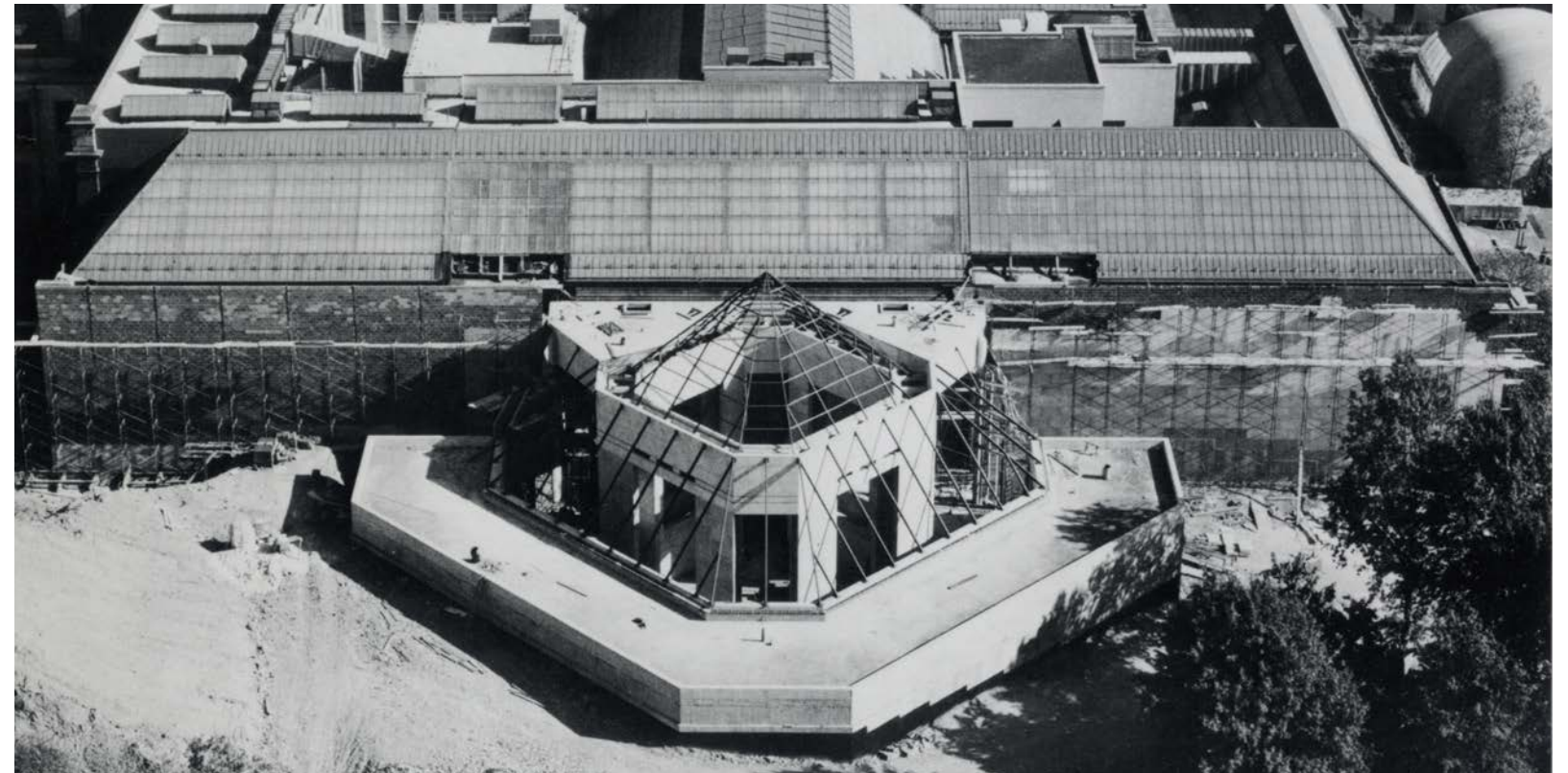
1970'S CONSTRUCTION OF LEHMAN WING AND STONE SCREEN WALL IN FRONT OF WINGS ABC FACADE
