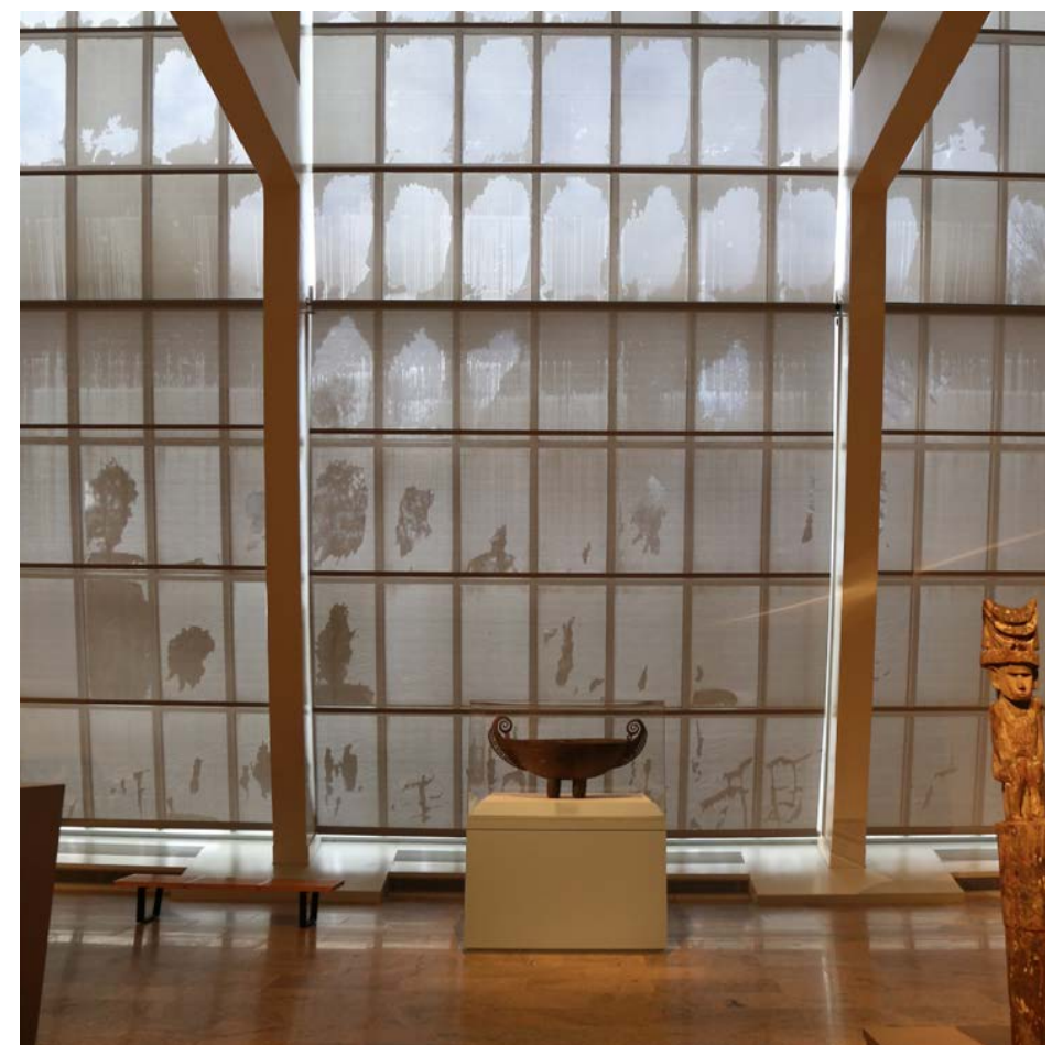
Interior: deteriorated film visible through mesh roller shades.
