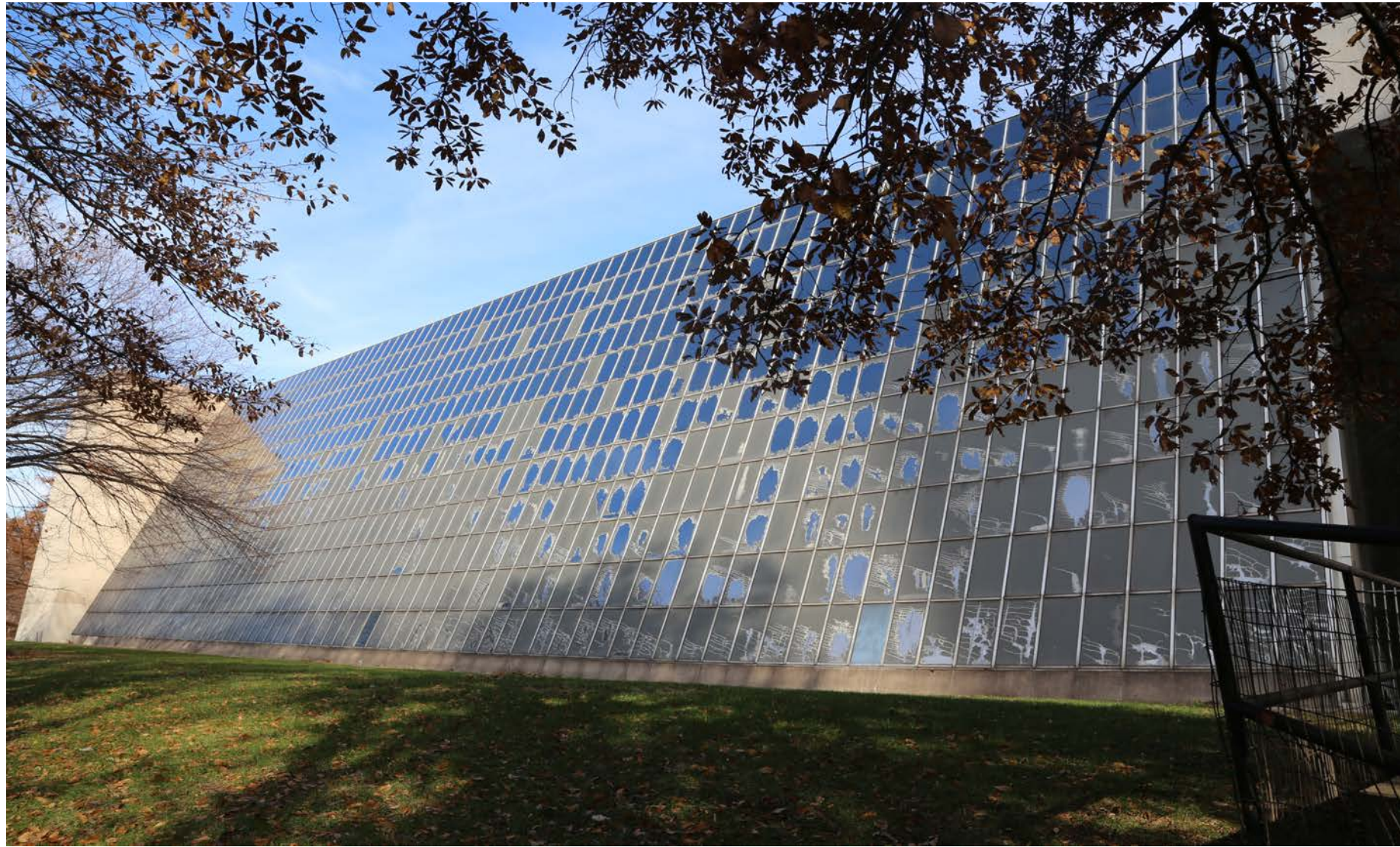
Existing Condition View from South of Rockefeller Sloped Glazing Sloped glazing is 200 feet long, 60 feet high and at a 70 degree slope with a surface area of approximately 12,000 square feet.
