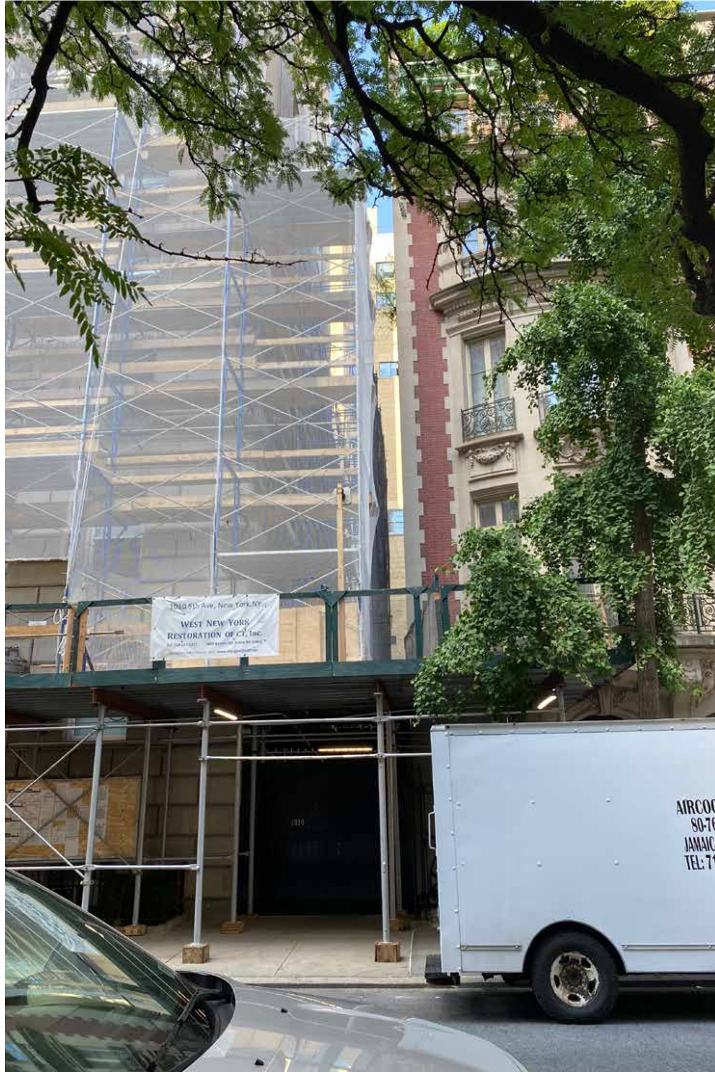
VP1 — View towards North from E82nd street (No's 1 and 3 E82nd street in view)
