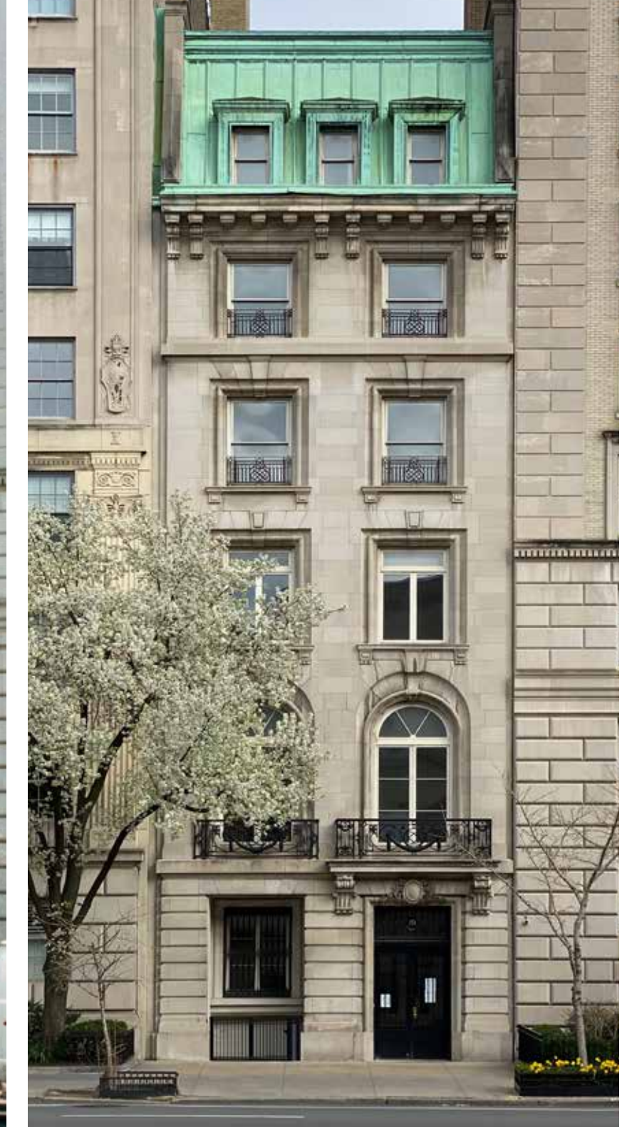
2021 — windows replaced in 90s following successful LPC application to match in kind original condition (reversing sash windows on L03 back to casement)
