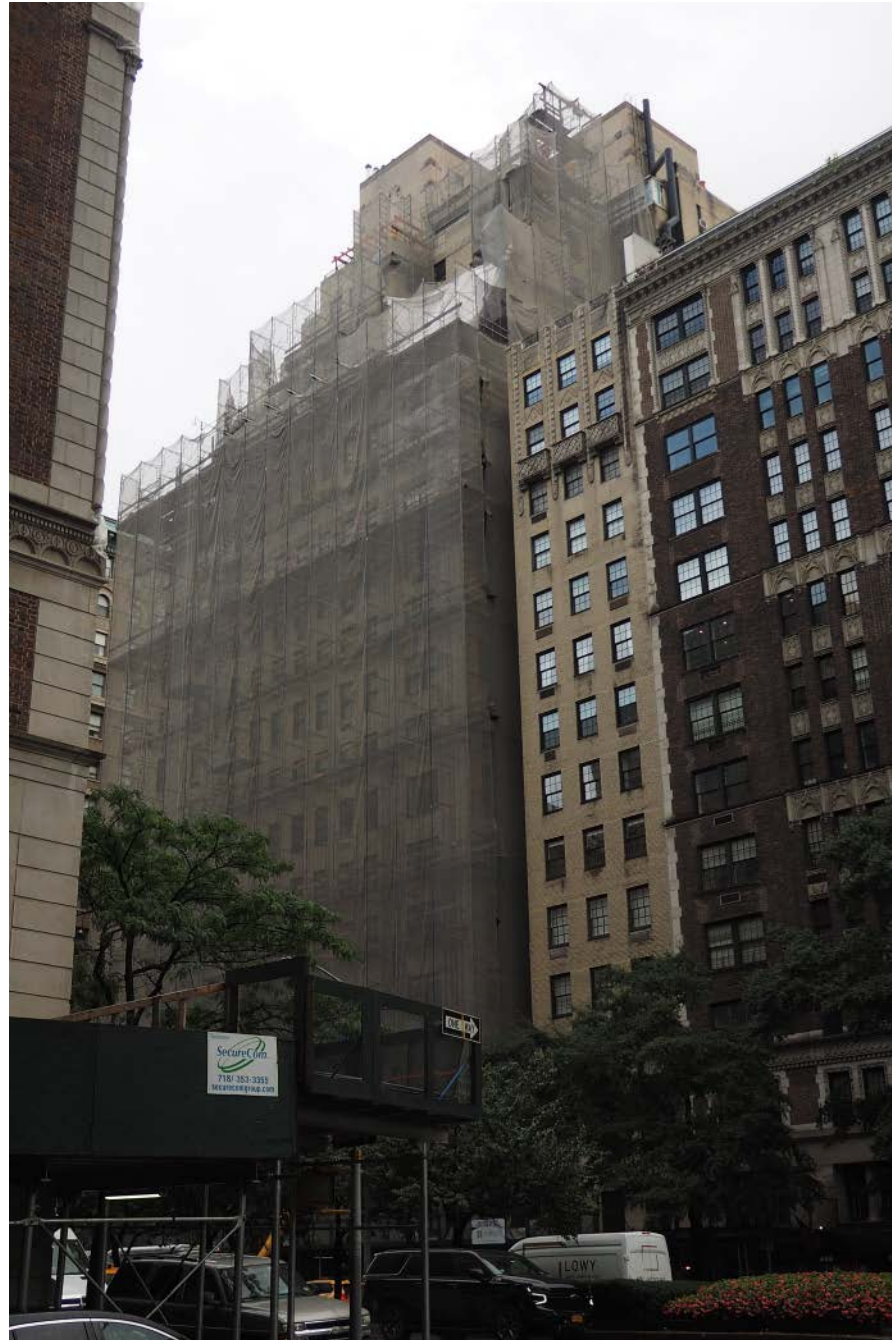
EXISTING ELEVATION WITH PERGOLA MOCK UP VIEW FROM PARK AVENUE & 78TH STREET
