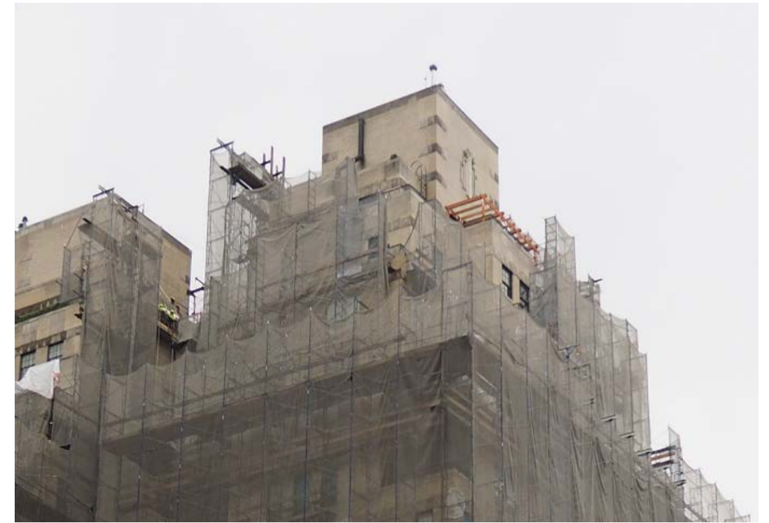
EXISTING ELEVATION WITH PERGOLA MOCK UP VIEW FROM PARK AVENUE BETWEEN 79TH AND 80TH STREETS
