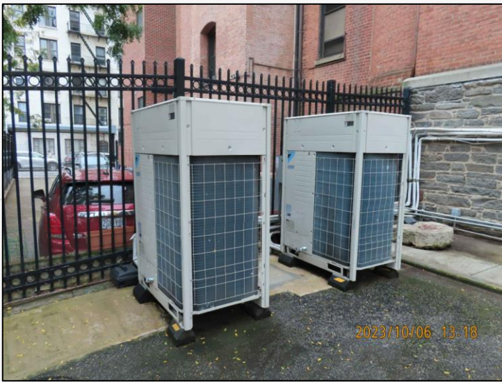
Existing HVAC Units
