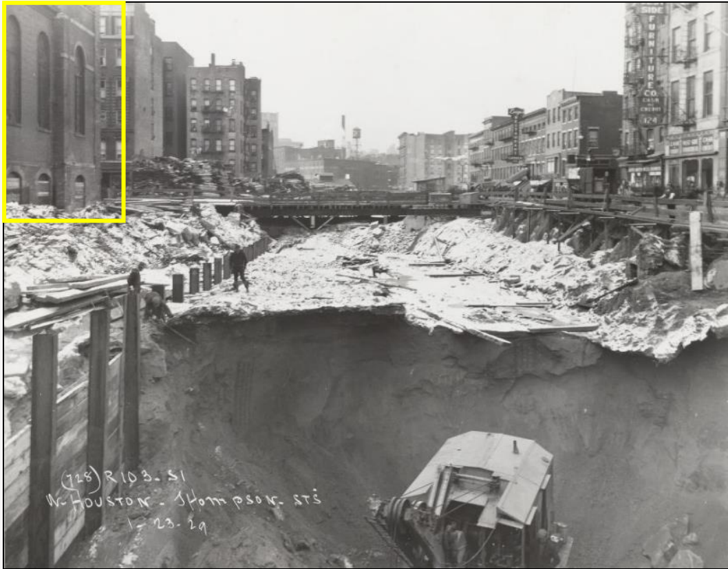
West Houston Street being widened to 6 lanes in early 1930's to accommodate new subway line. Multiple buildings on either side of the street were demolished for the street.
