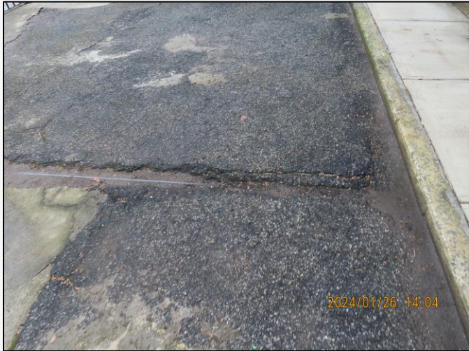
Existing courtyard pavement showing cracks
