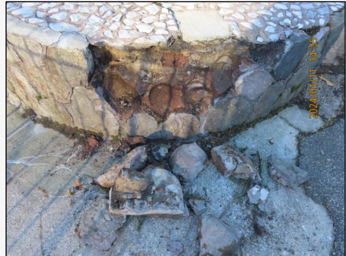
Closeup of the base damage
