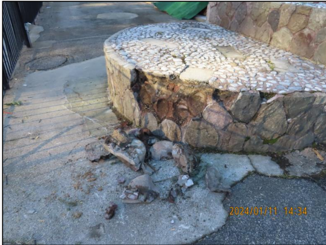
Existing Fatima Statue Base Damaged
