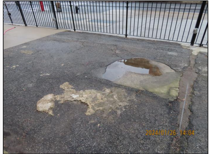
Existing courtyard pavement with potholes
