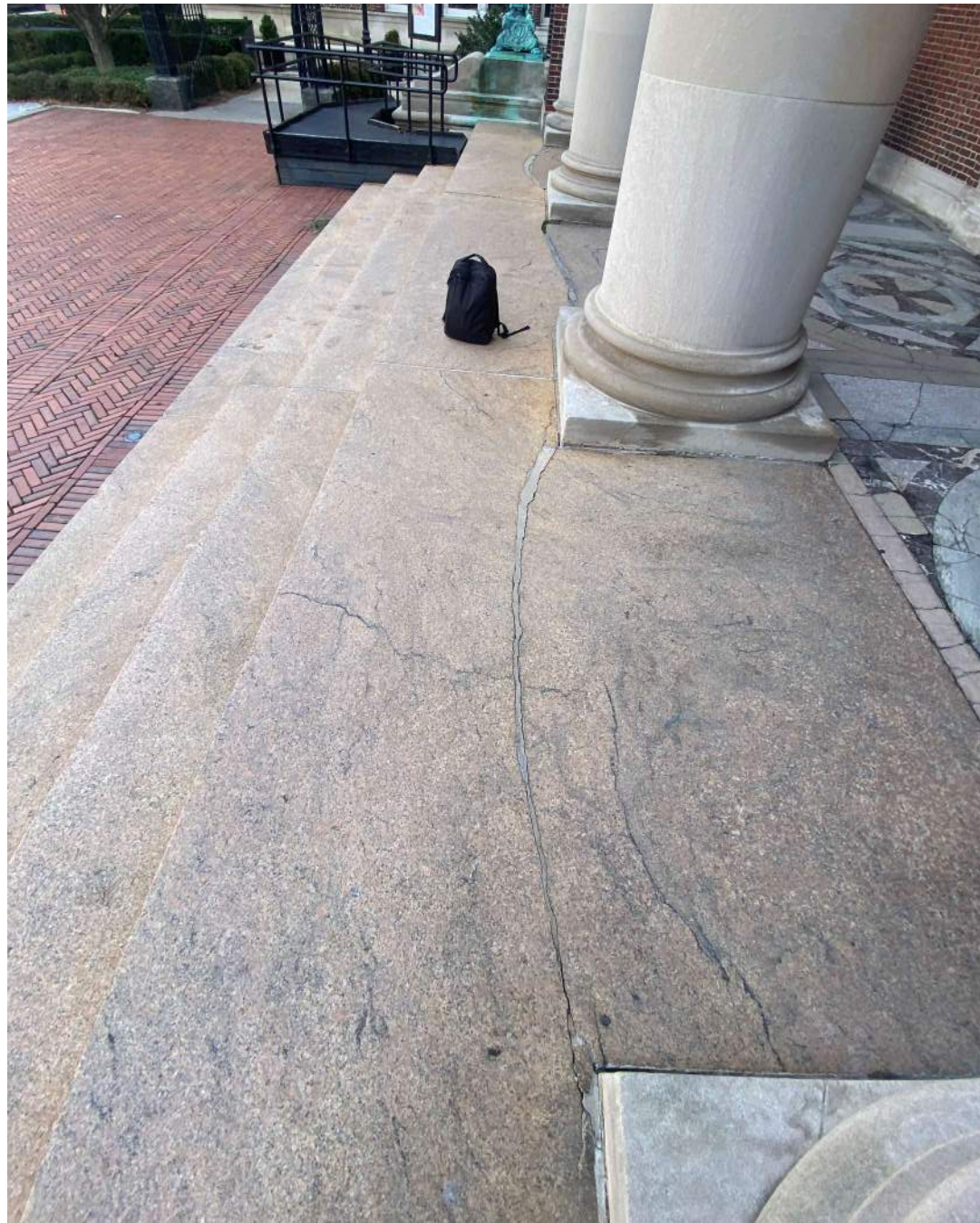
NORTH-SOUTH CRACK FULL LENGTH OF CHAPEL ENTRANCE STEPS.
