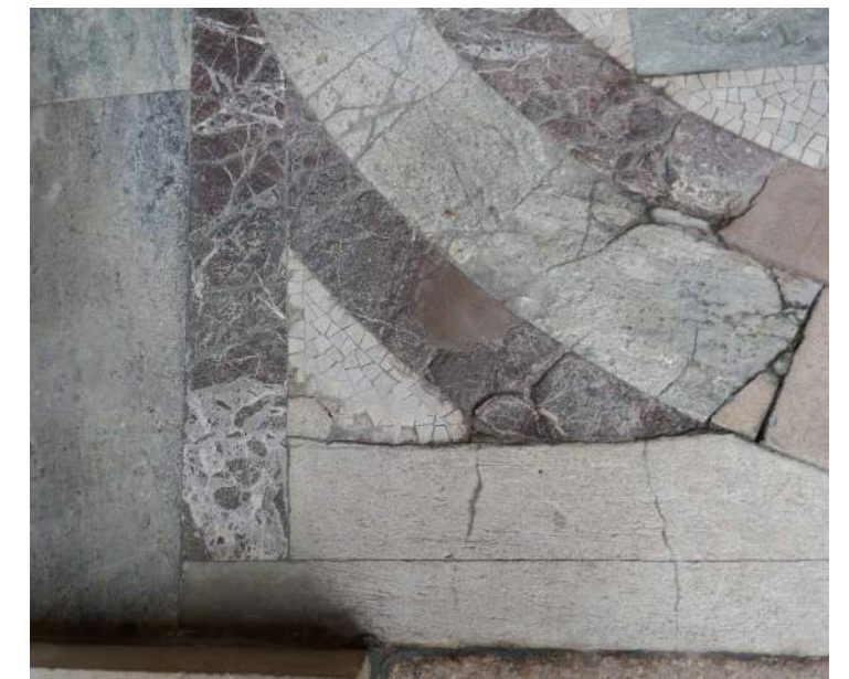
SOUTHERN BAY WITH BADLY DAMAGED AND REPLACED STONE
