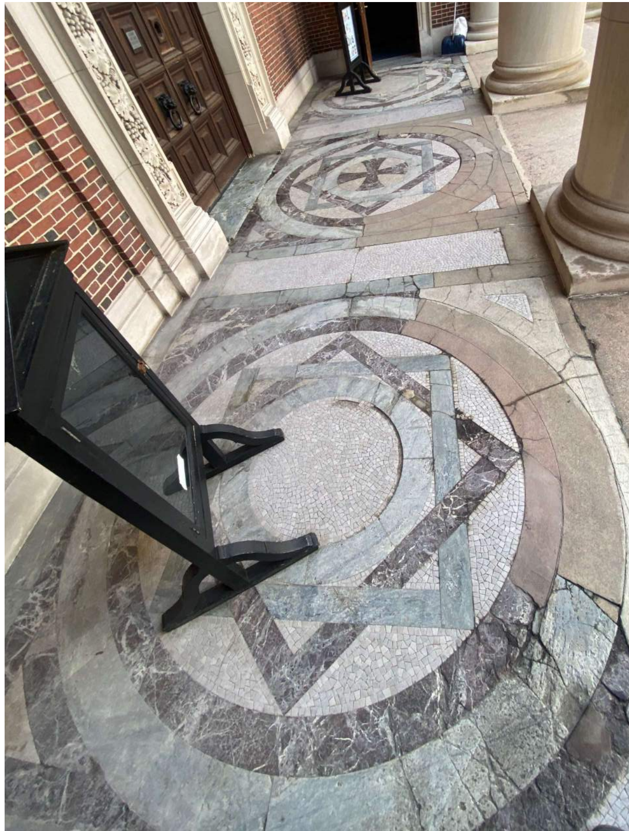
LOOKING SOUTH - DAMAGED AND REPLACED PAVING
