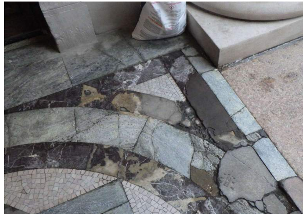
SOUTHERN BAY WITH BADLY DAMAGED AND REPLACED STONE
