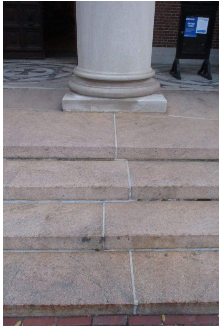
OPEN BED JOINTS AT CHAPEL ENTRANCE STEPS.
