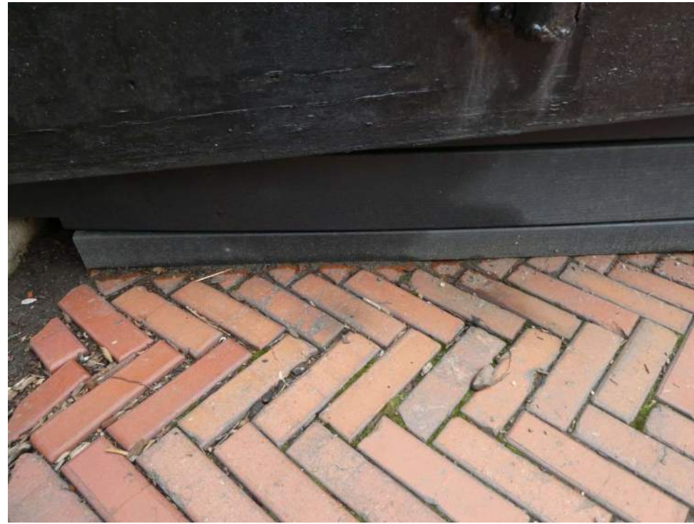
PLAZA AT EXISTING RAMP WITH HEAVING AND ERODED JOINTS.
