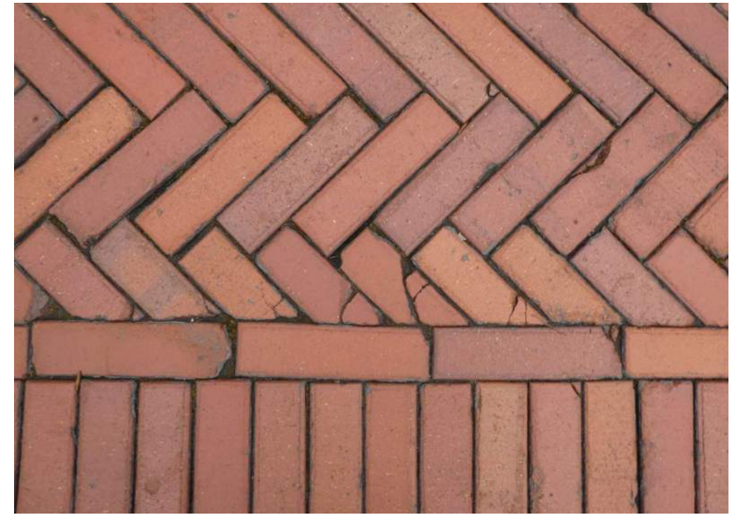
BRICK PAVERS - CRACKED BRICK, HEAVING AND ERODED JOINTS
