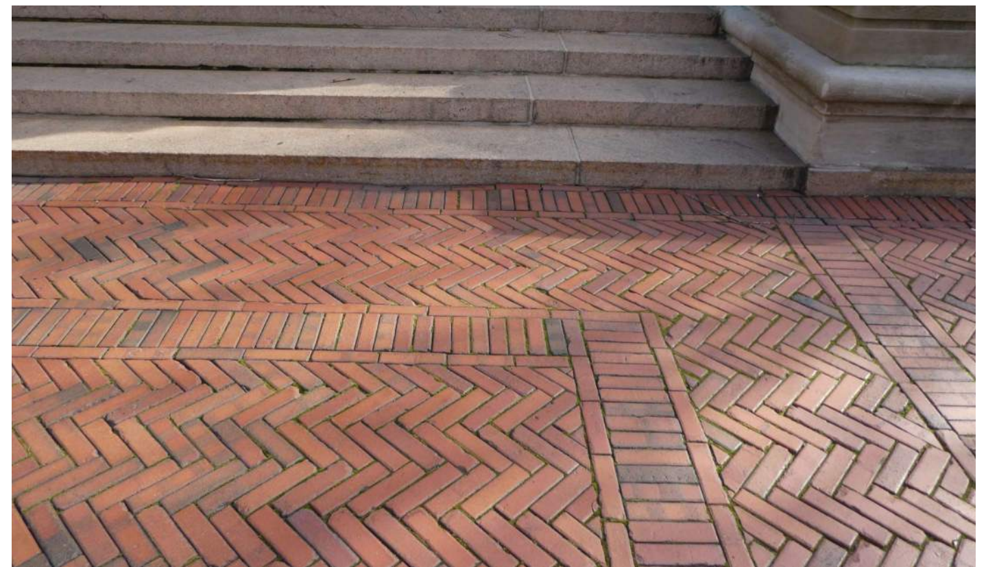
SOUTHEAST CORNER WITH HEAVING AND ERODED JOINTS.
