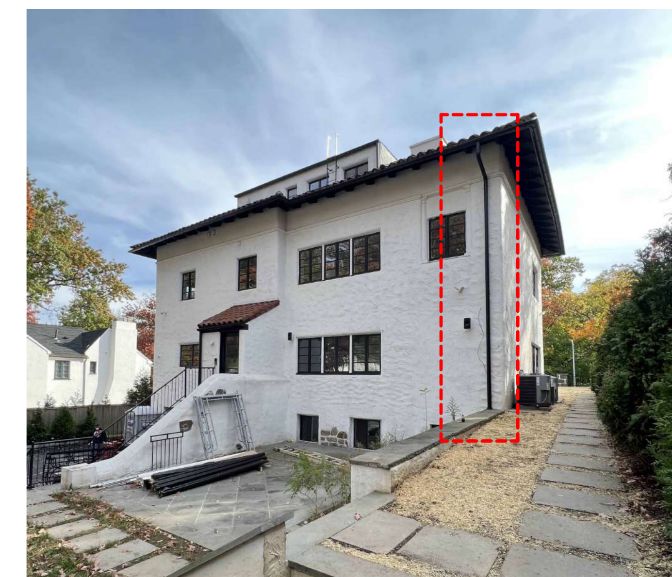
(2) EXISTING ALUMINUM GUTTER
