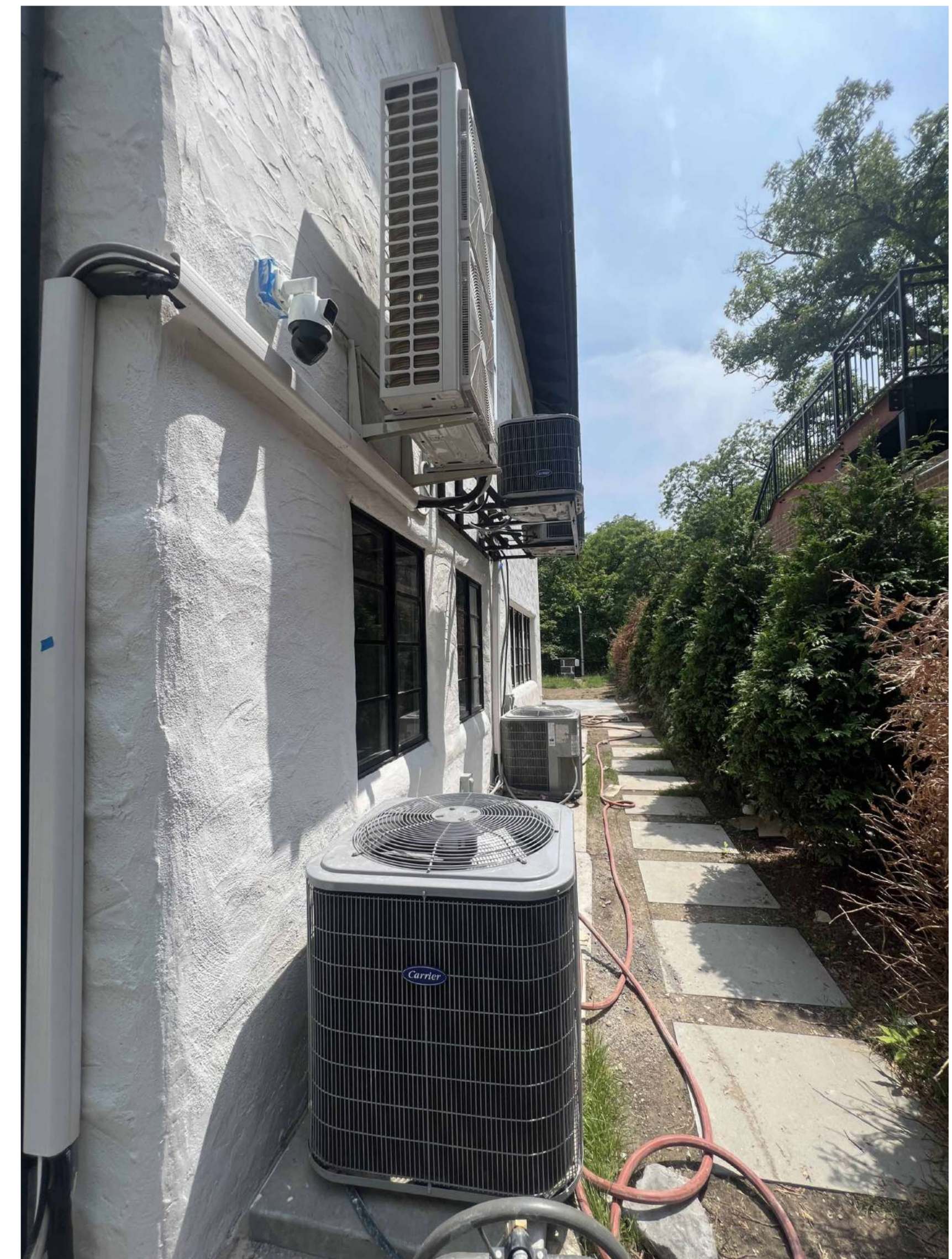
WEST FACADE CAMERA AND HVAC EQUIPMENT
