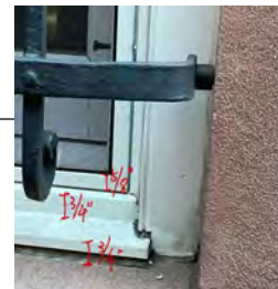
CLOSE-UP PHOTO OF WOOD BRICK MOLD. OUR INTENTION IS TO MATCH THIS DETAIL
