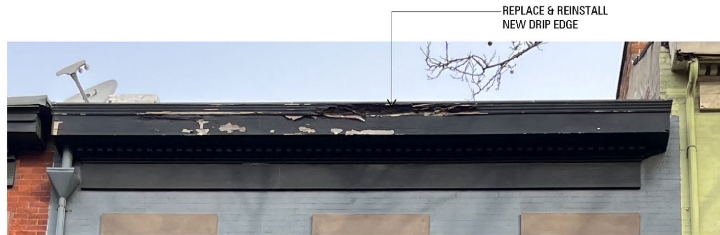
3. DETERIORATING SECTION OF CORNICE TO BE REPAIRED
