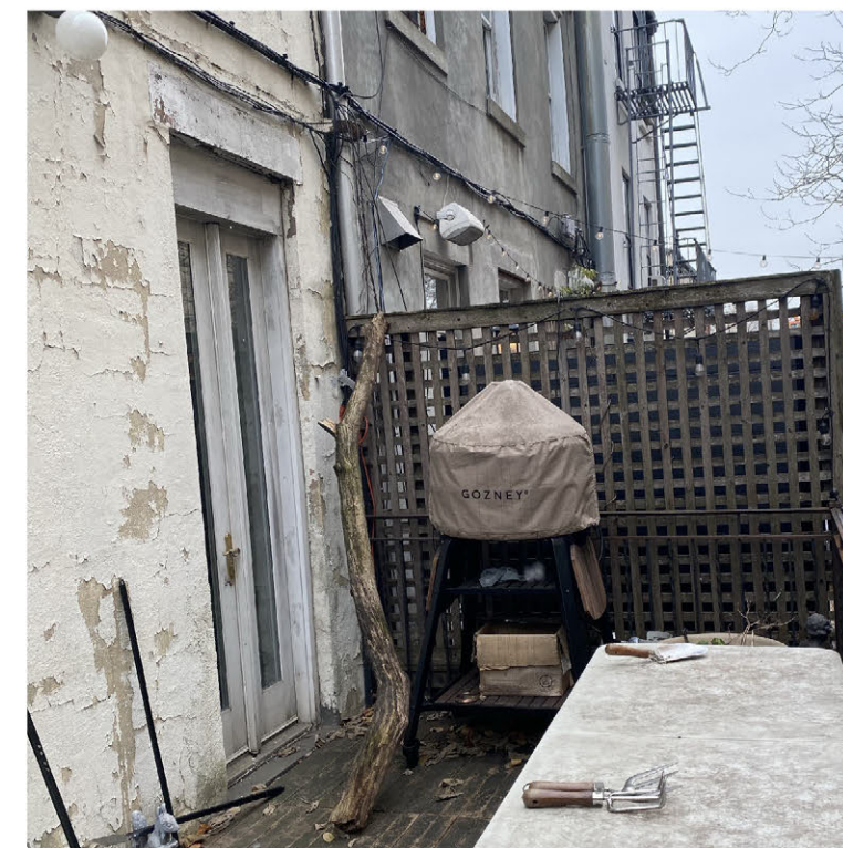
3. EXISTING DOUBLE HUNG NON-ORIGINAL FRENCH CASEMENT DOORS AT 1ST FLOOR IN POOR CONDITION
