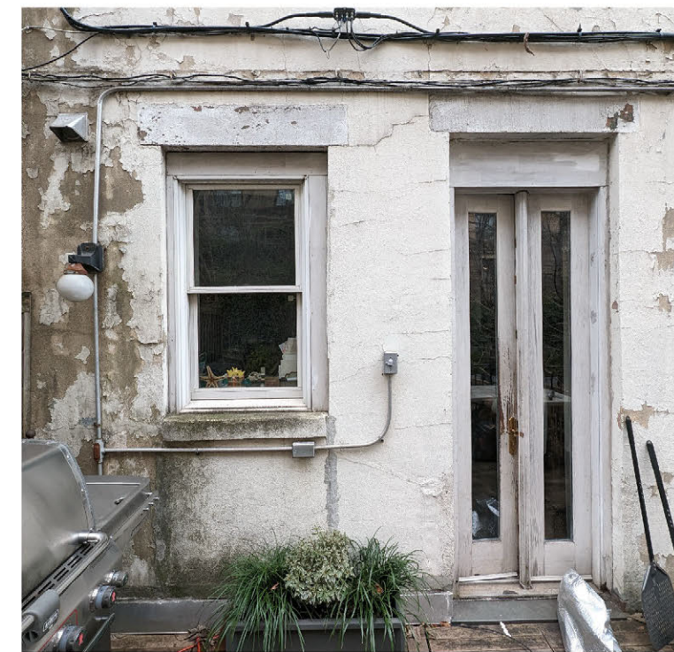
2. EXISTING DOUBLE HUNG NON-ORIGINAL WINDOW & FRENCH CASEMENT DOORS AT 1ST FLOOR, ALL IN POOR CONDITION
