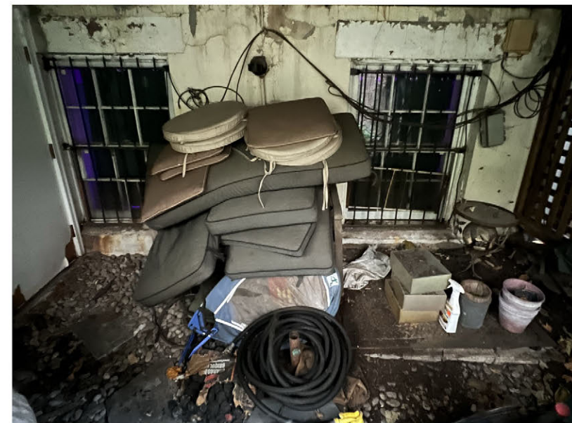
4. EXISTING SIX-OVER-SIX NON-ORIGINAL WINDOWS, ALL IN POOR CONDITION
