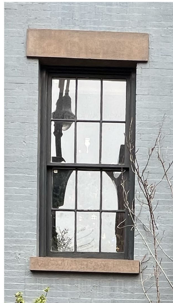
1. EXISTING SIX-OVER-SIX NON-ORIGINAL WINDOWS, TYP
