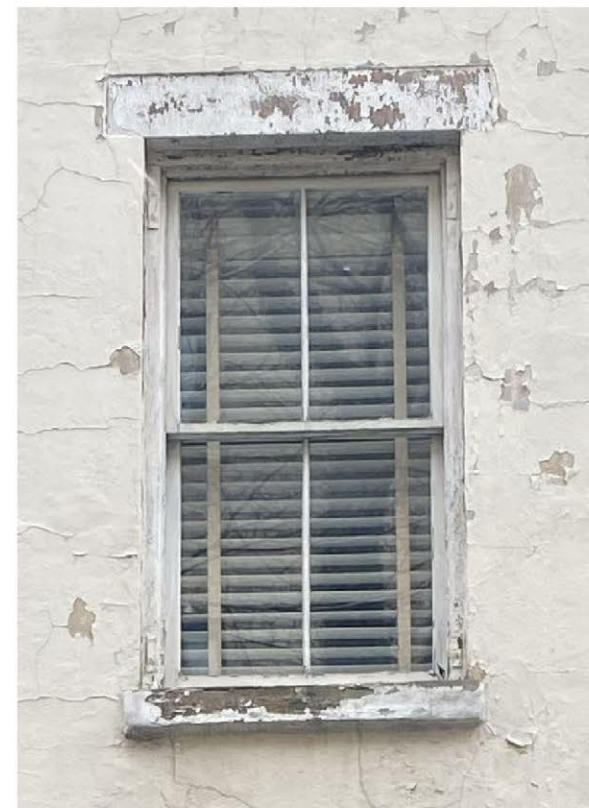
2. EXISTING TWO-OVER-TWO NON-ORIGINAL WINDOWS, ALL IN POOR CONDITION
