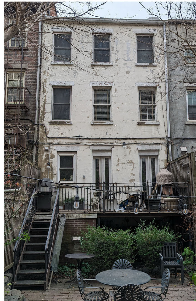
1. EXISTING REAR FACADE IN POOR CONDITION
