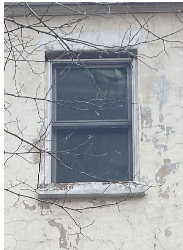
1. EXISTING DOUBLE HUNG NON-ORIGINAL WINDOWS, ALL IN POOR CONDITION
