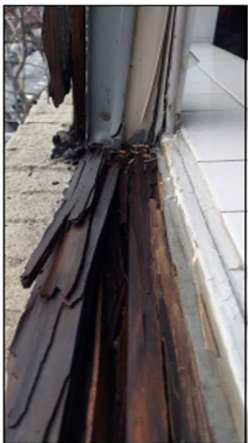
DETERIORATING WINDOW SILL
