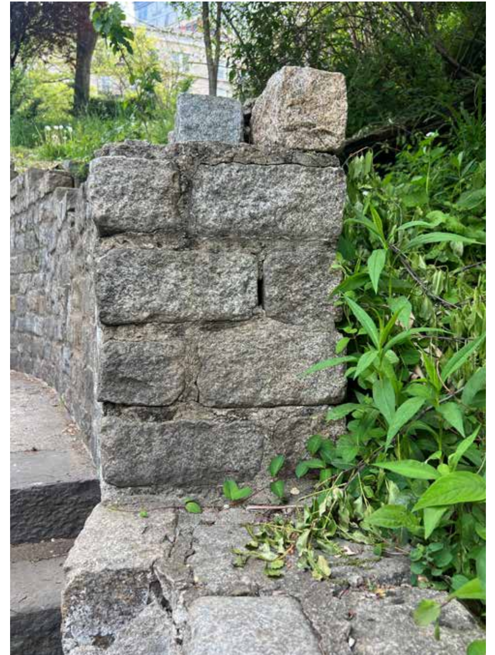
1966 wall overlaps treads by 1-3 granite blocks. Existing wall is 16" wide. No coping allows water in the joints and poor base is causing granite blocks to separate.
