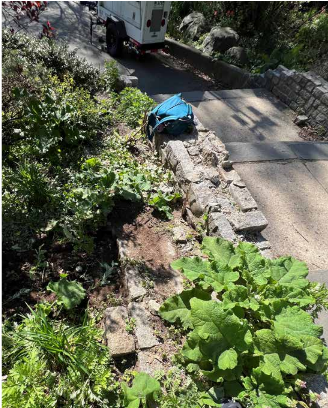
Overgrown swale on the left. 1966 cheekwall was built on top of pre-1964 cheekwall wall but also overlapping the treads, narrowing the stairways.
