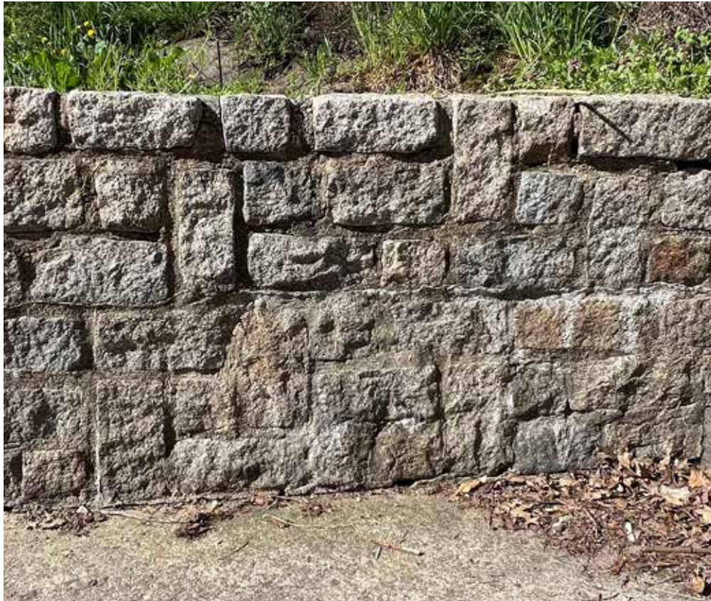
Existing granite block- to be cut thinner and re-used as facade, both sides, in the same layout as existing pattern
