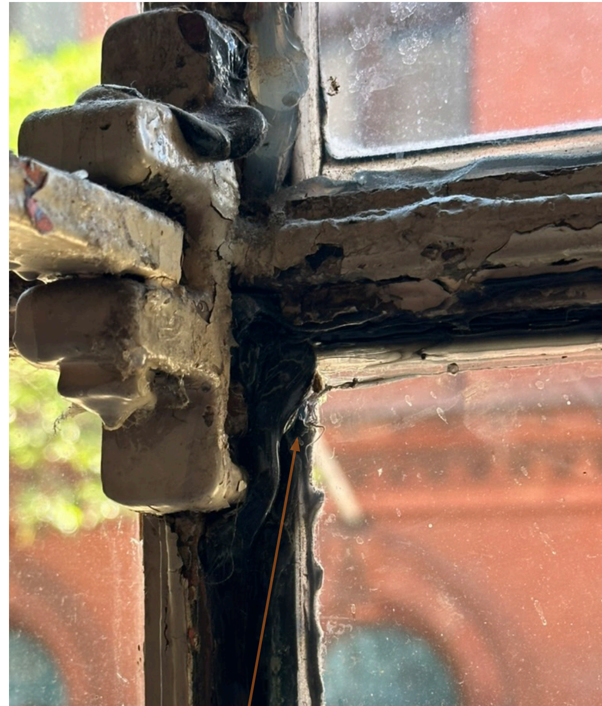
Window frame stops missing and replacement glass is caulked in
