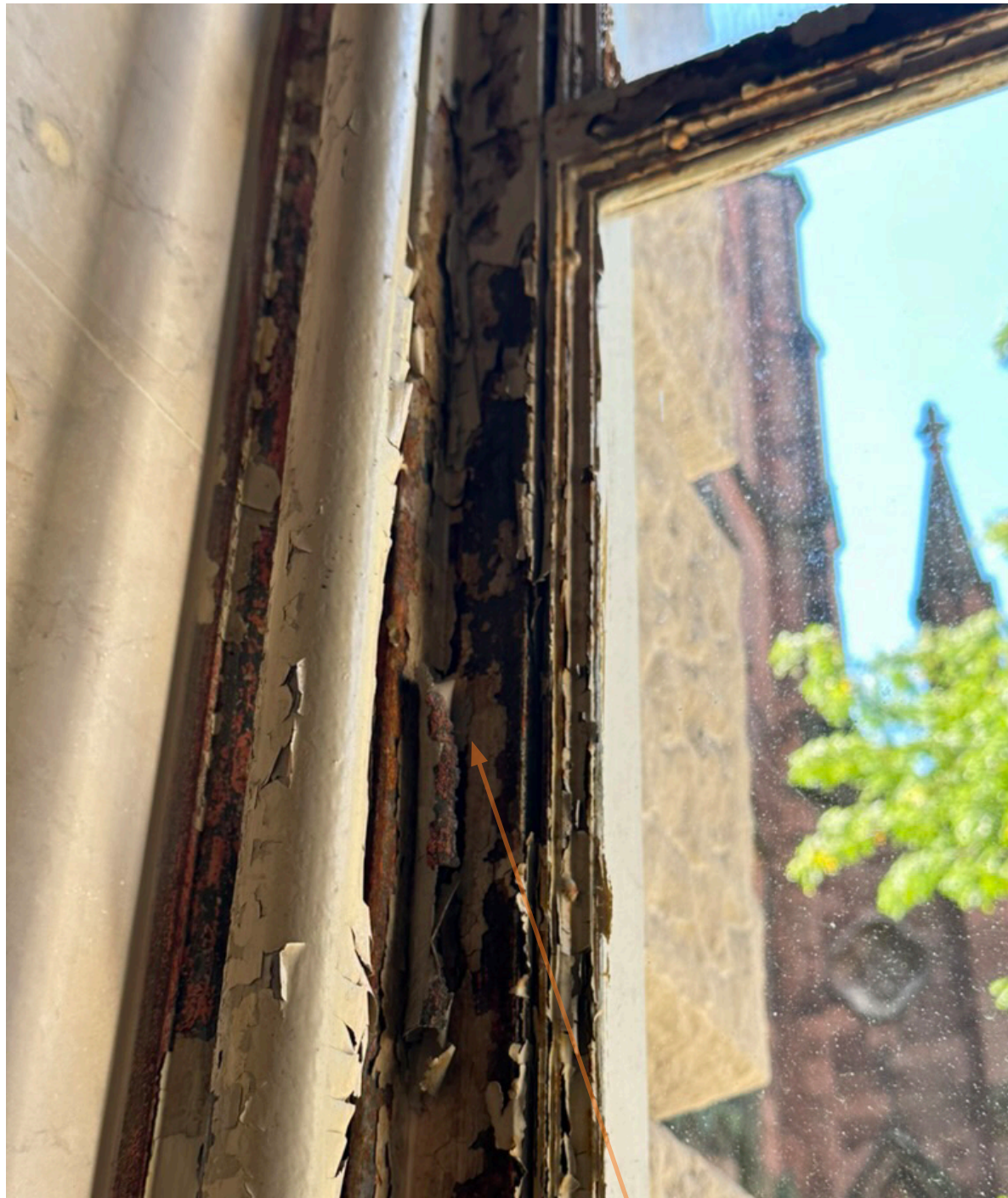
Windows 5, 6, 7 with severe paint peeling and corrosion
