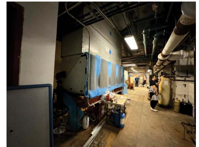
EXISTING SOUTH COOLING TOWER TO BE REMOVED
