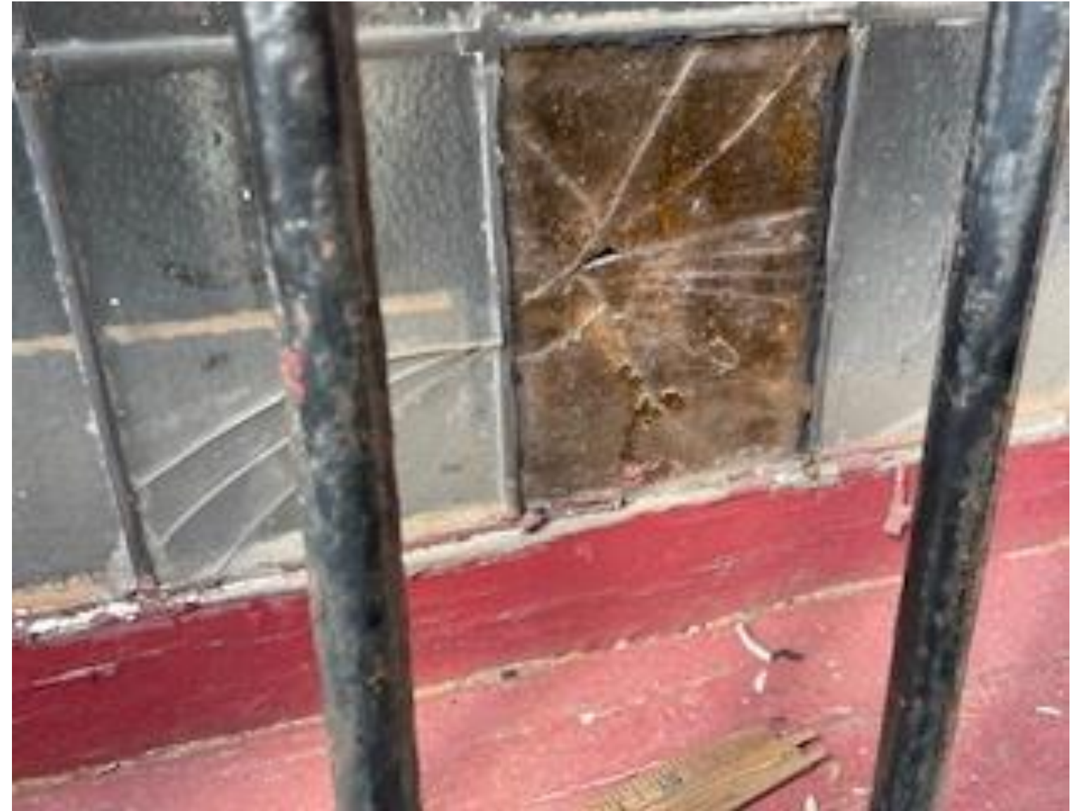
Detail of Condition – Right Basement Window
