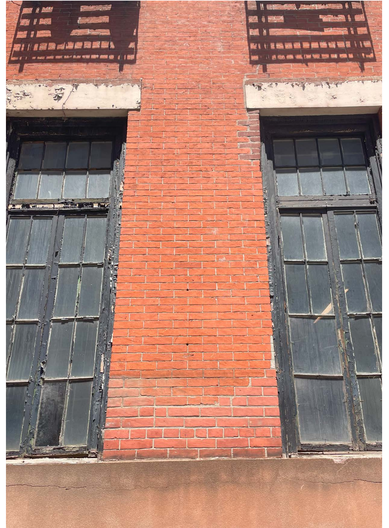
CURRENT BRICK CONDITION IS VERY POOR
