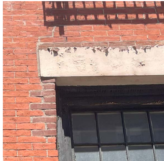
3. Lintels are in poor condition with the existing paint peeling
