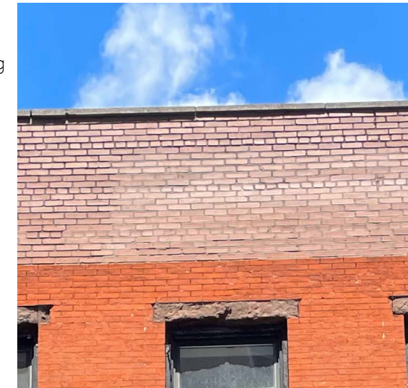
4. Parapet built with insensitive materials
