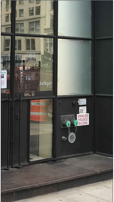
Opaque glass covering pipe chase on Storefront #2.
