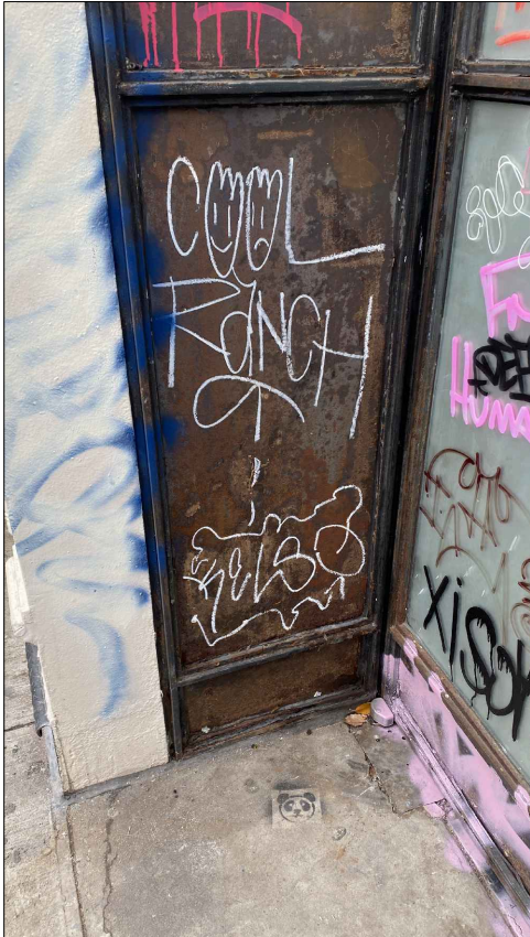
Tags and graffiti, broken glass, rust and delaminating in existing doors on Storefront #3.
