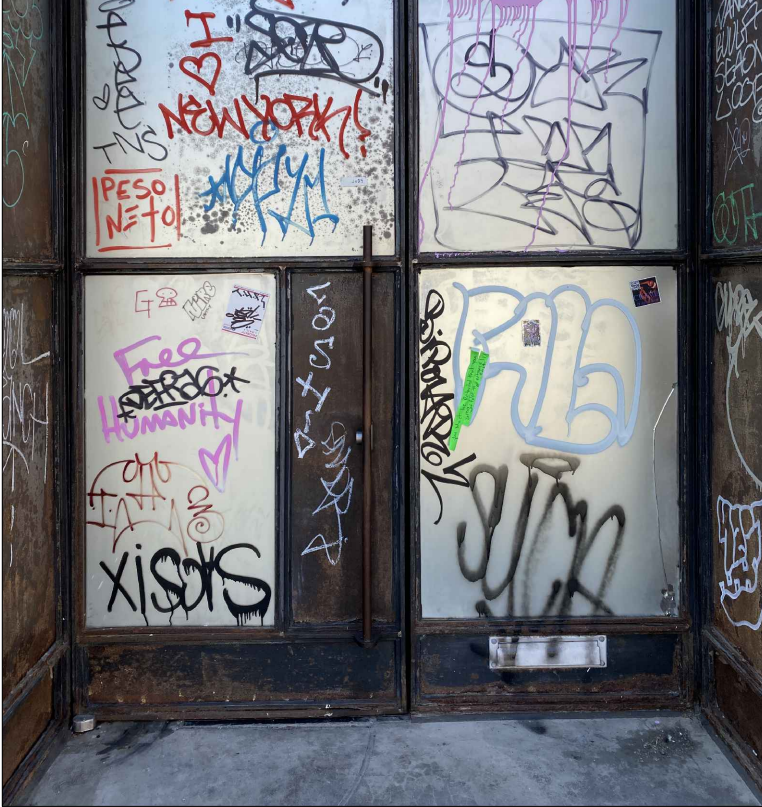
Vandalized glass door. Graffiti and broken glass. Rusted frames.
