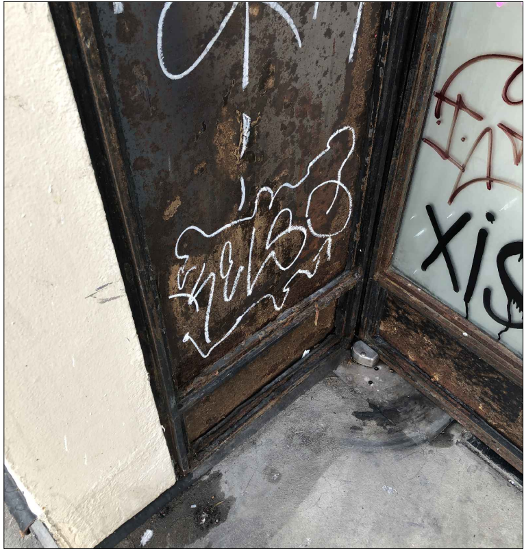
Rust and delamination on side panels.
