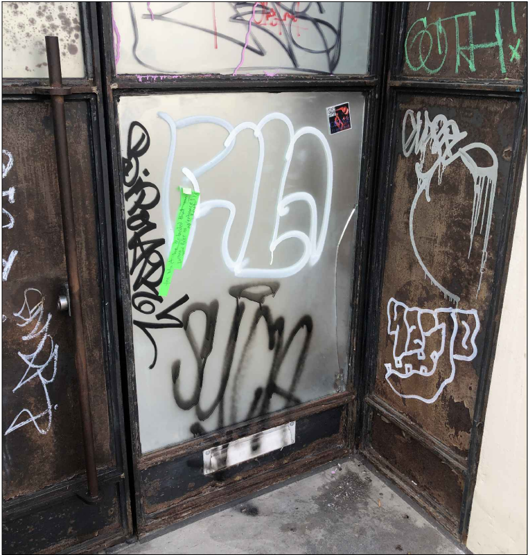
Rust and delamination on metal doors, broken glass.
