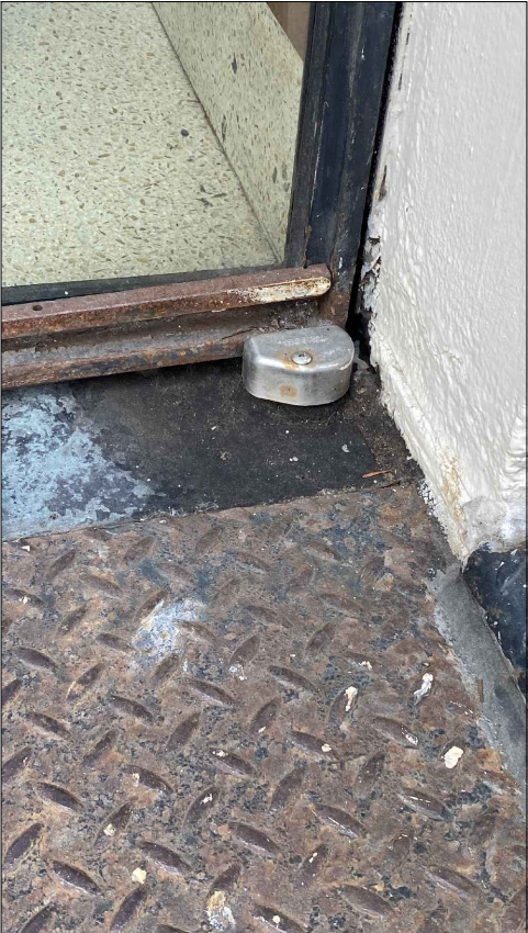
Deteriorated window and rail on Storefront #4.
