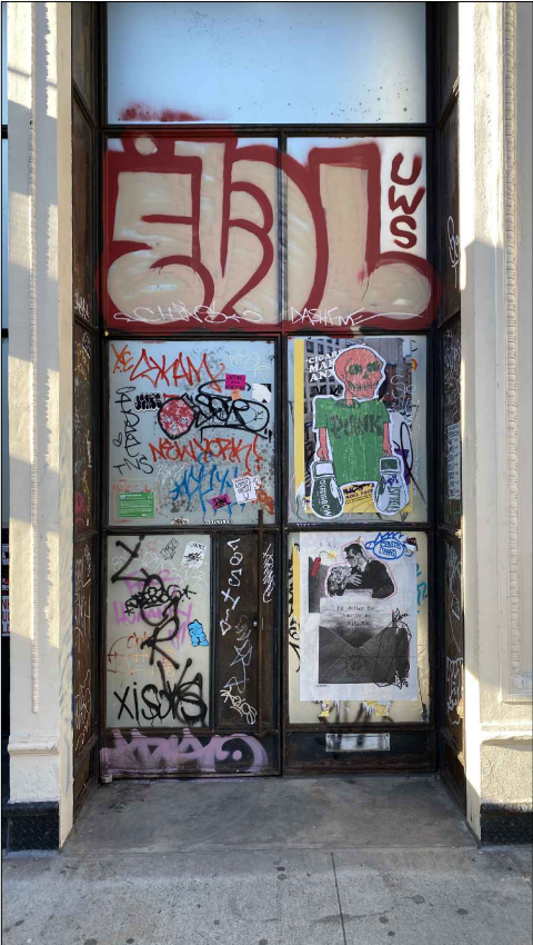
Tags and graffiti, broken glass, rust and stickers on Storefront #3.
