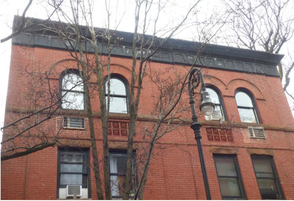
Third floor and cornice, with missing terra-cotta spandrels.
