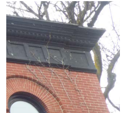
Existing Cornice To Be Repaired/Repainted
