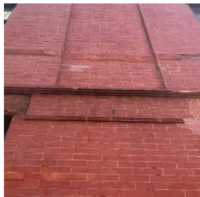
Masonry/Brick Courses To Be Restored
