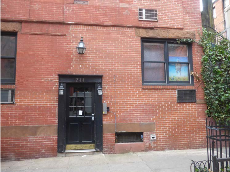
Through-wall louvers have been installed throughout the front facade and the stoops and areaway was removed.
