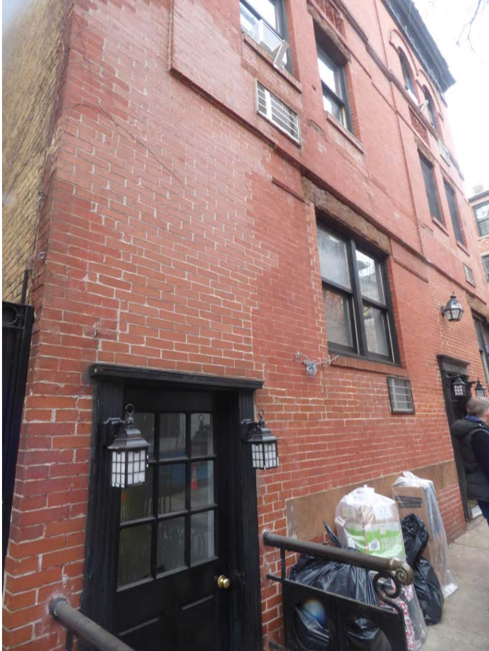
The stoops were removed and window openings were modified; non-matching brick infill was installed.
