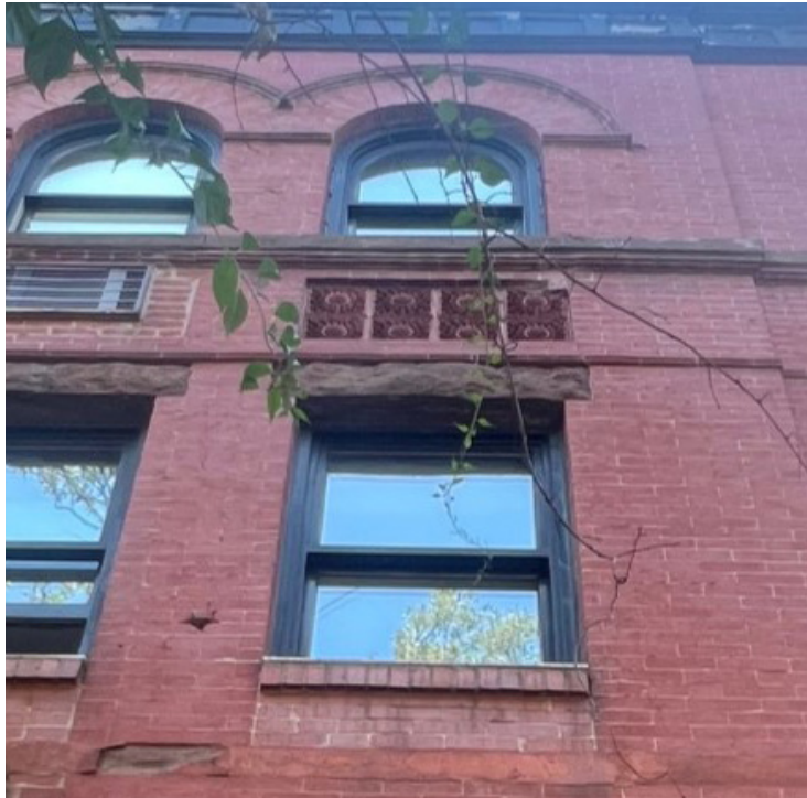
Existing Brick Sills and Damaged Masonry Courses
