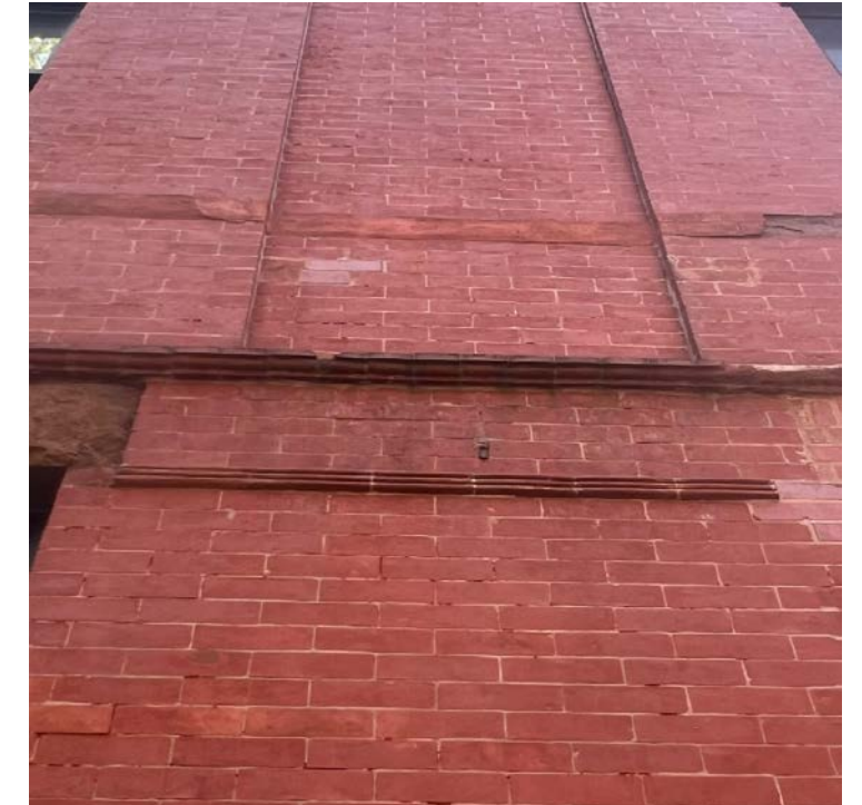
Broken Masonry Courses
