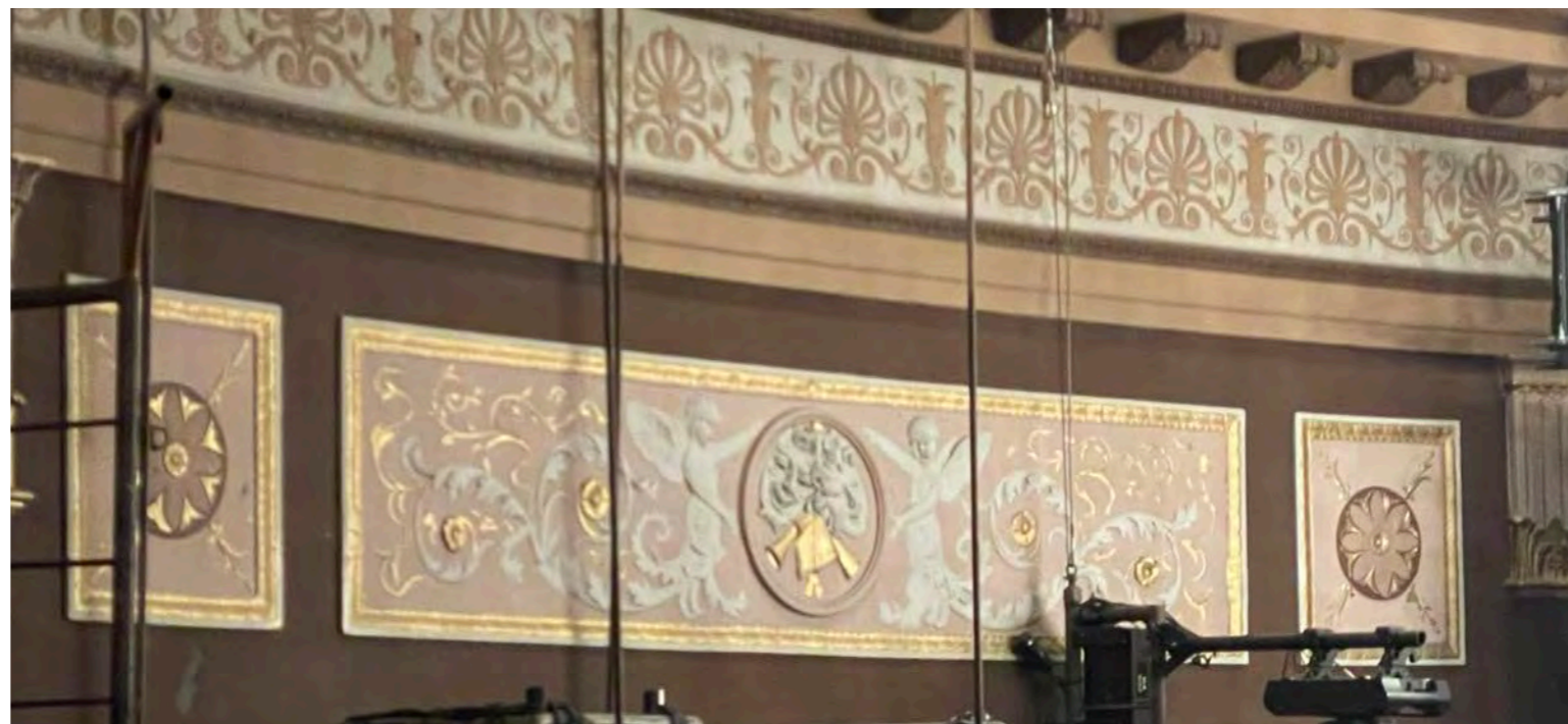
Panel detail above house left boxes
