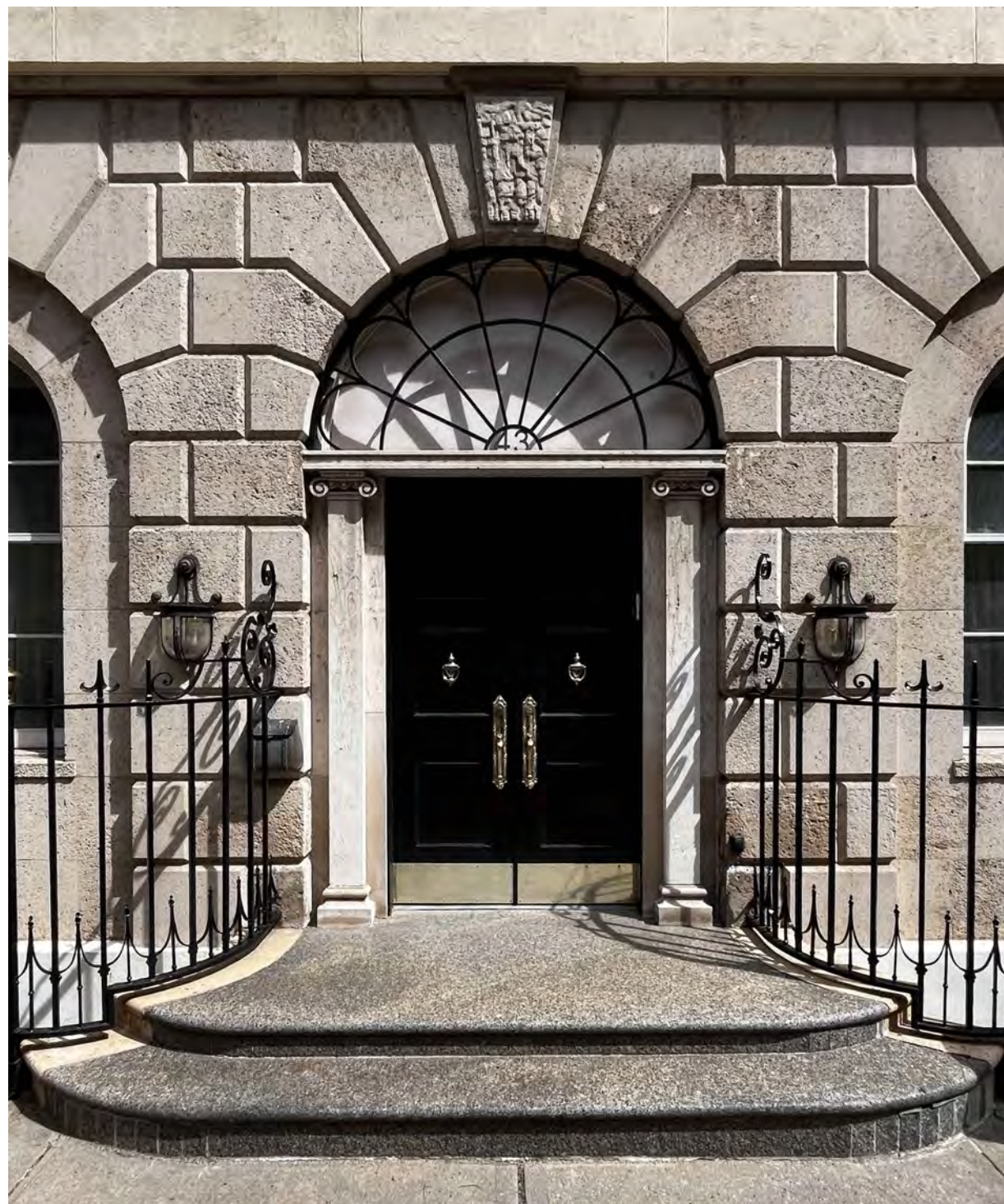
43 EAST 70TH STREET: EXISTING ENTRY DOOR
