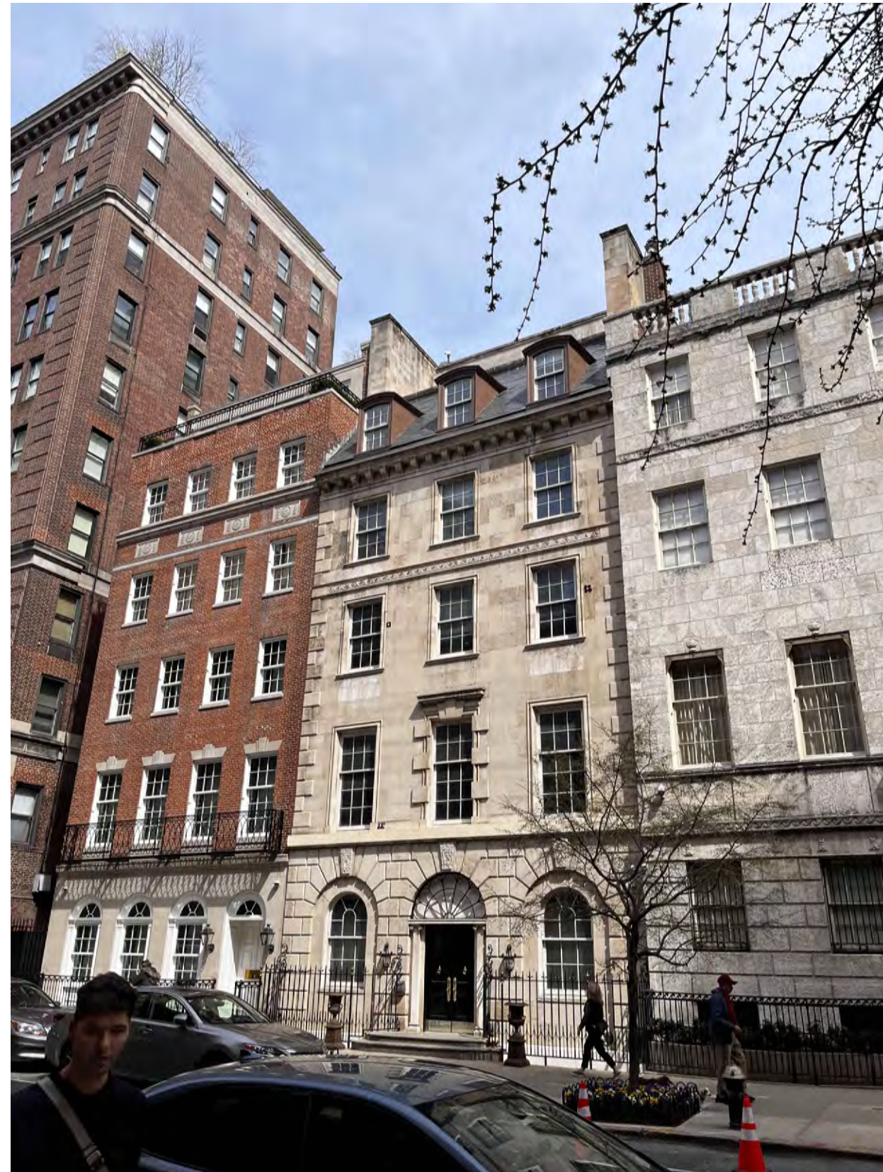
41-43 EAST 70TH STREET: SOUTH FACADE EXISTING CONDITIONS
