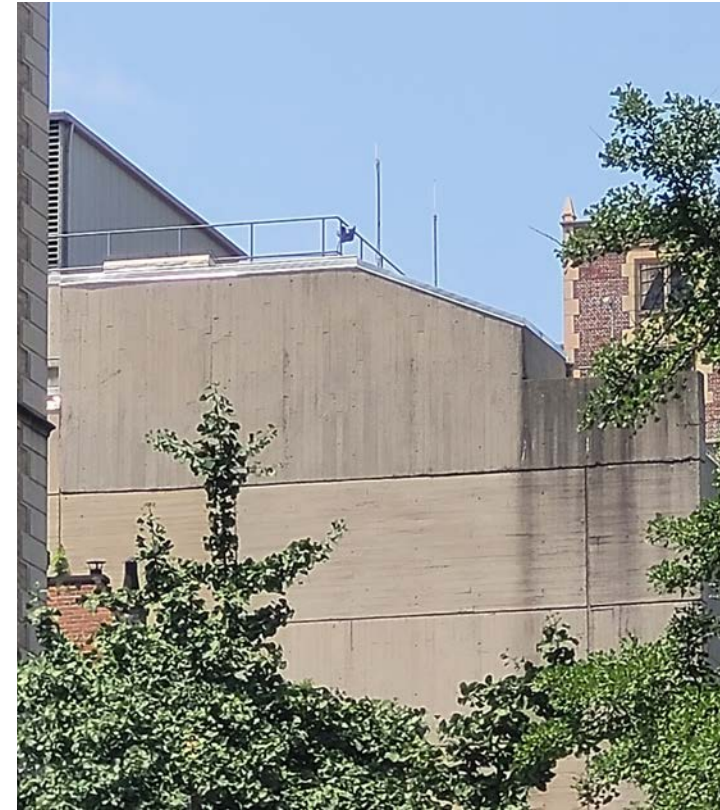
East party wall and bulkhead from 75th St. (facing west) Photograph by: PBDW Architects
