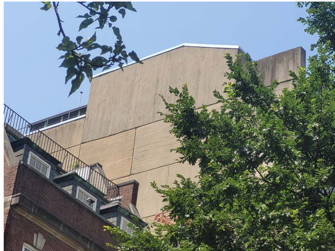
East party wall from 75th - enlarged (facing west) Photograph by: PBDW Architects
