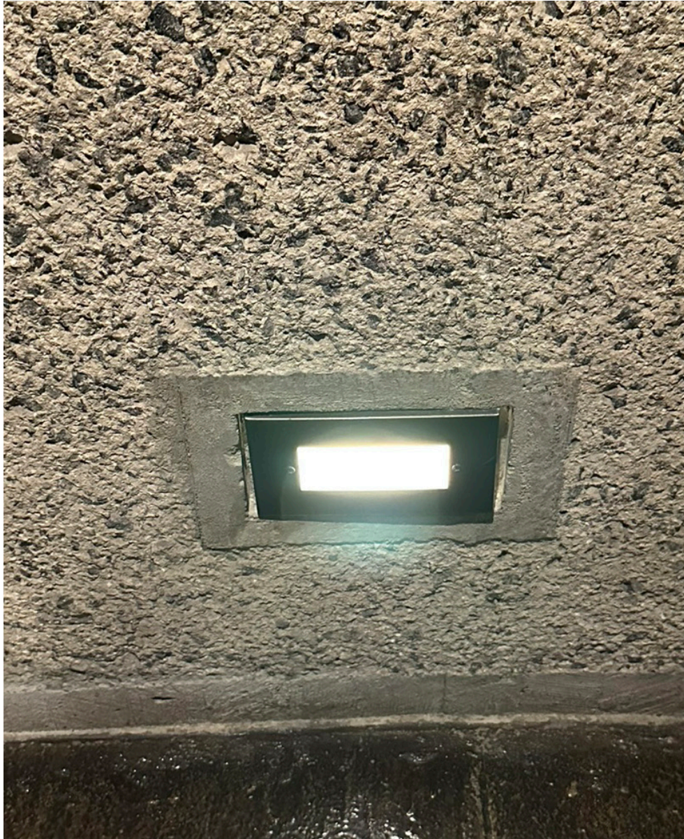
Light fixture insert at stairs
