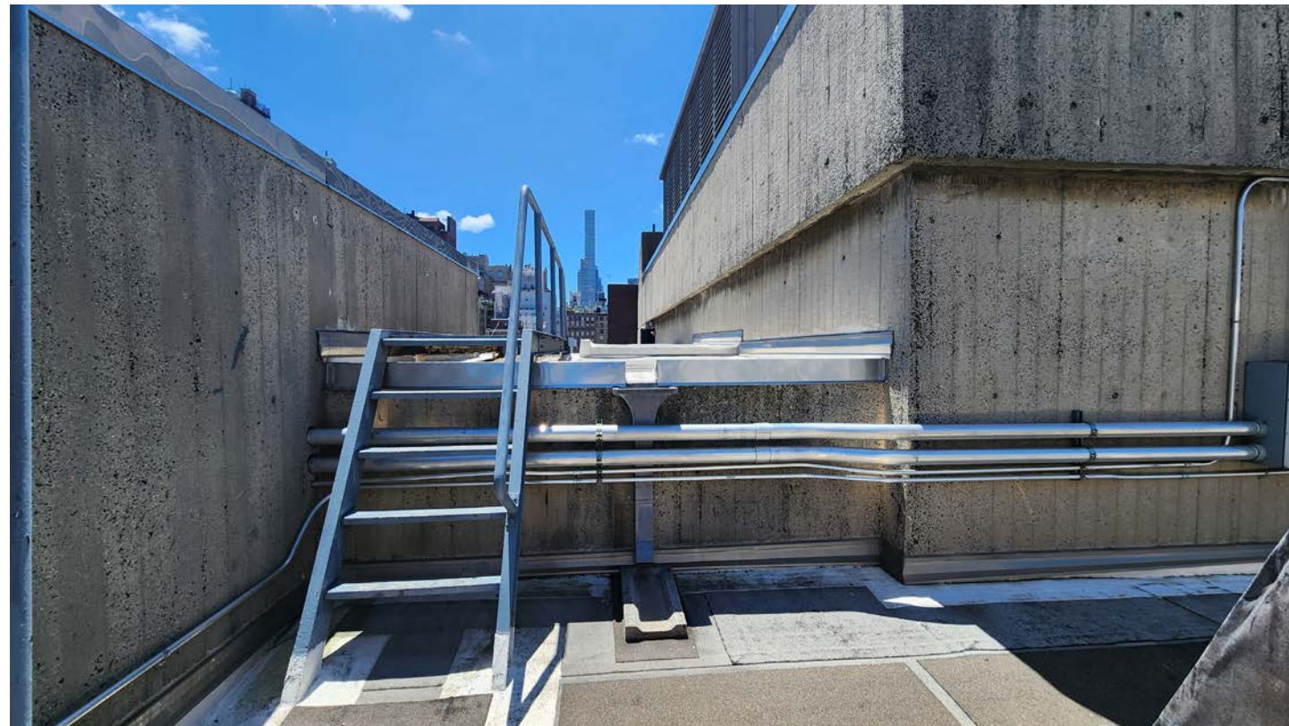
4: Stair bulkhead + bridged connection to mechanical penthouse (facing south) Photograph by: Herzog & DeMeuron
