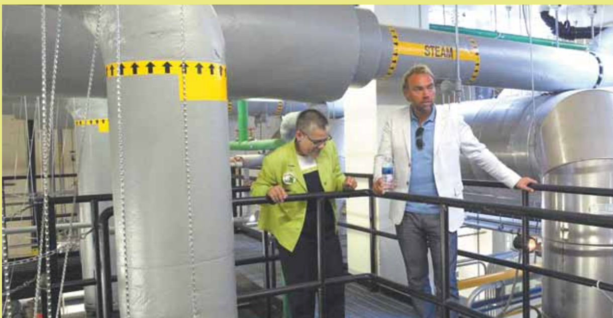
NYCHA Board Member Margarita López shows Johan Ernst Nilson, known as 'Johan the Explorer,' the boiler room at Castle Hill Houses in the Bronx. Mr. Nilson is travelling from the North Pole to the South Pole to raise awareness of environmental sustainability.
