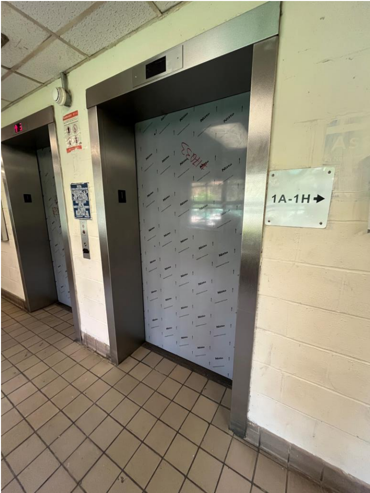
New elevators at Union Avenue Consolidated
