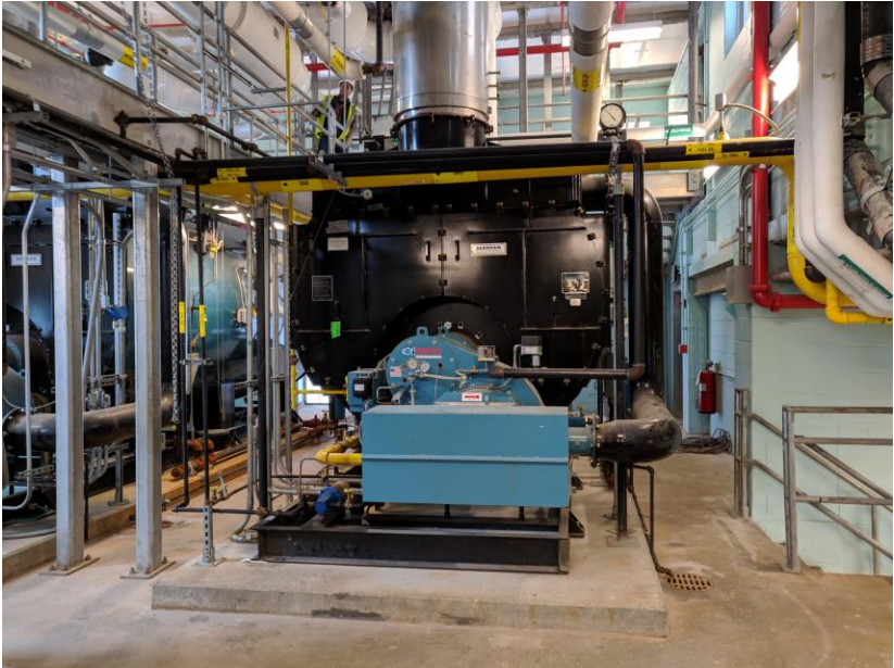
New boilers at Coney Island Houses
