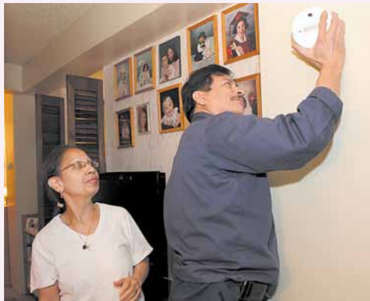
Queensbridge South resident Elizabeth Crespo watches NYCHA Maintenance Worker Roberto Balina install a new carbon monoxide alarm in her apartment on April 25, 2012.
