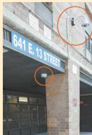
Shown in the circles are two of the new closed circuit security cameras installed at Campos Plaza.
