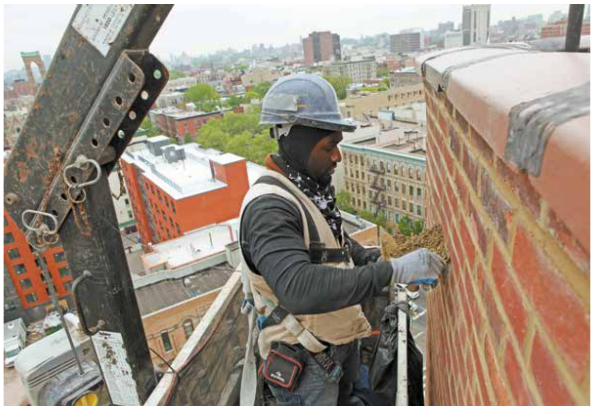
The money NYCHA received from the federal government will be used for capital improvements, including exterior brick work.
