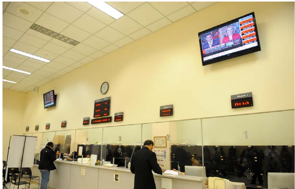
Queuing System Displays and Monitors behind Counter at 9 Metrotech
