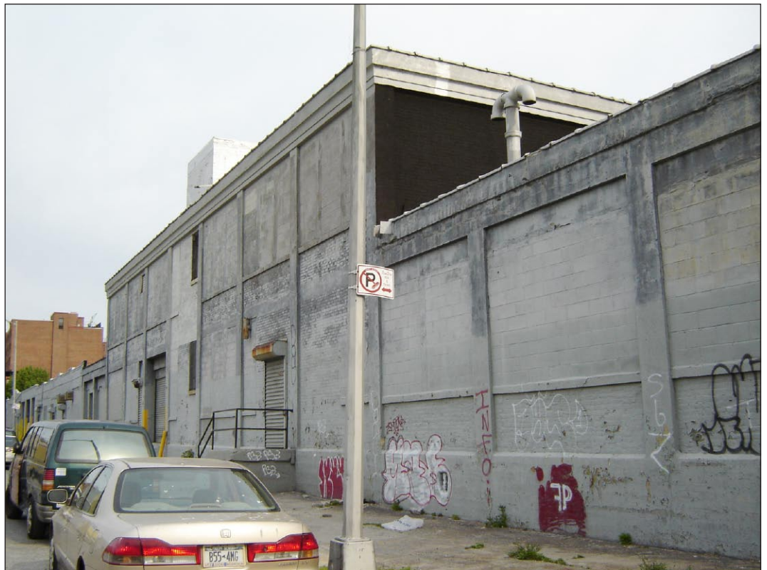
View from First Street and the west side of the Gowanus Canal, looking northwest towards Building 3 on the project site.
