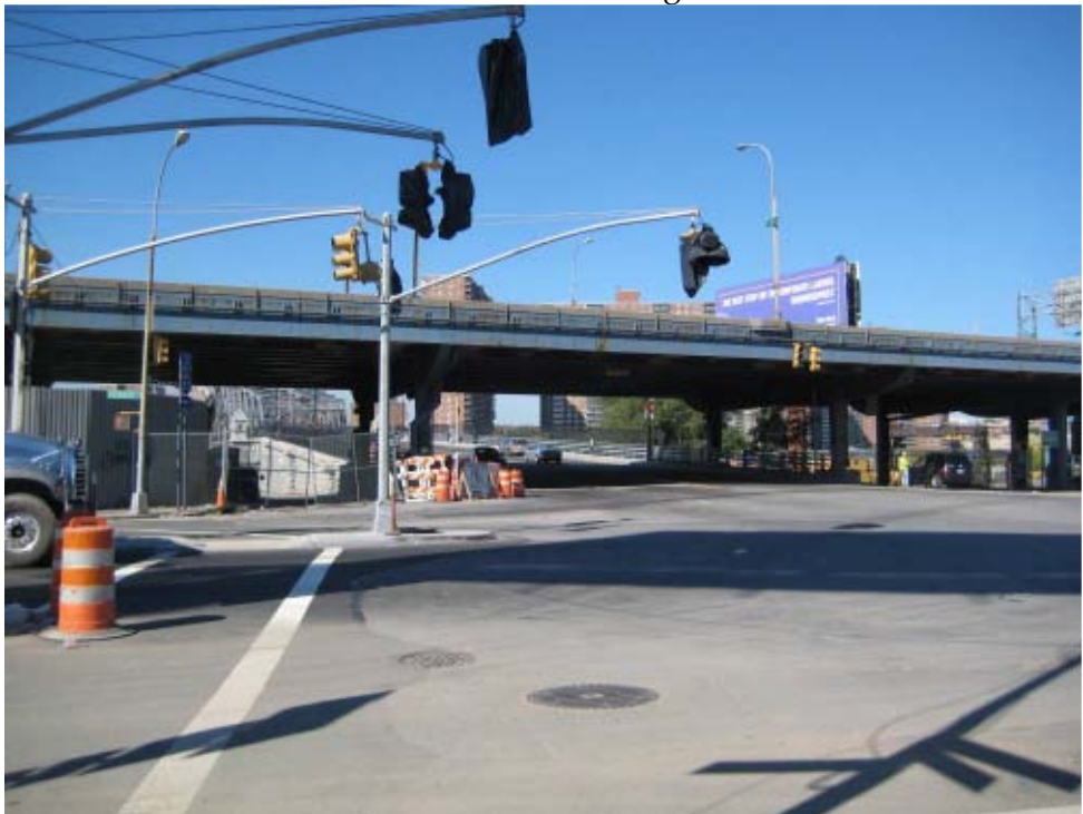
(8) Major Deegan Expressway and 145 th Street Bridge viewed looking west from East 149 th Street.
