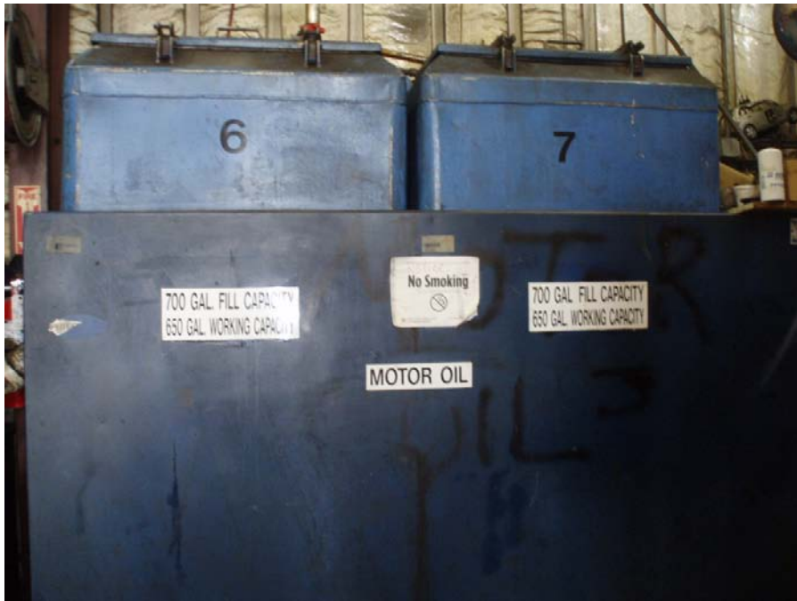
Photograph 3 – Lot 100: Two 700-Gallon Above Ground Storage Tanks
