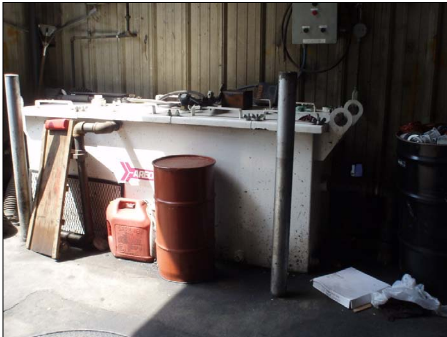
Photograph 10 – Lot 100: Oil/Water Separator
