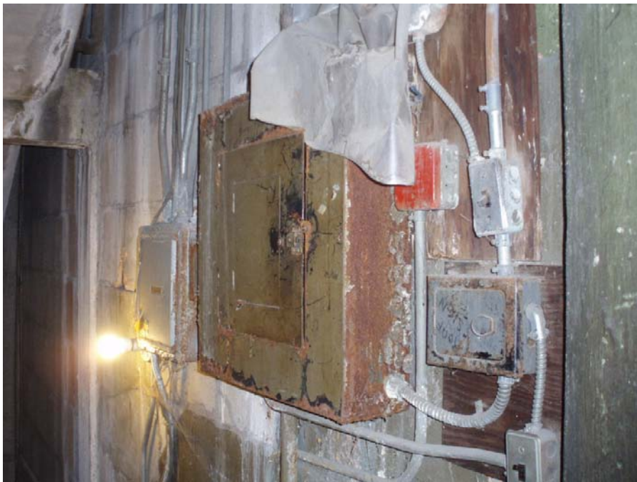
Photograph 40 – Lot 107: Electrical Equipment
