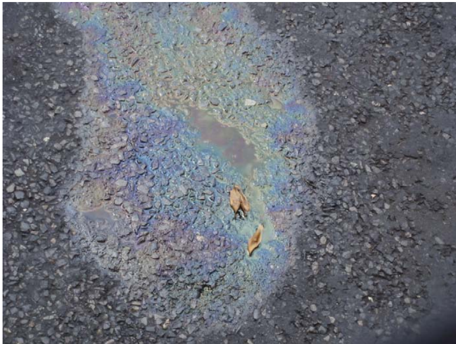
Photograph 12 – Lot 100: Sheen on Water Near Garage Bay Entrance
