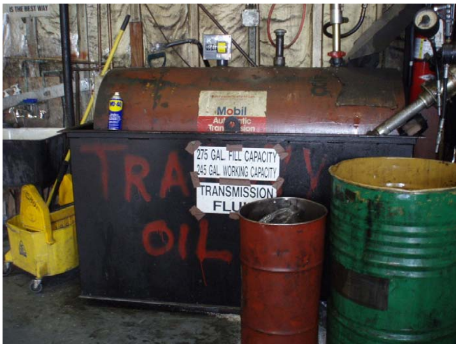
Photograph 4 – Lot 100: 275-Gallon Above Ground Storage Tank
