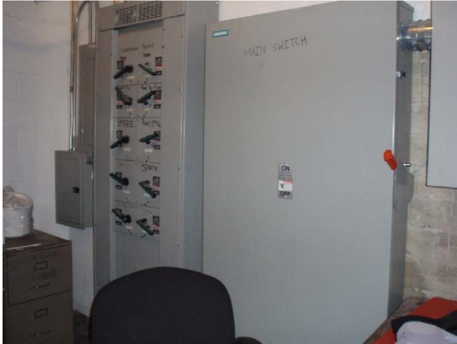
Photograph 33 – Lot 103: Electrical Equipment
