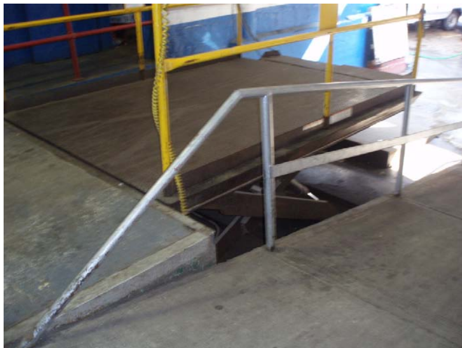
Photograph 28 – Lot 103: Hydraulic Lift
