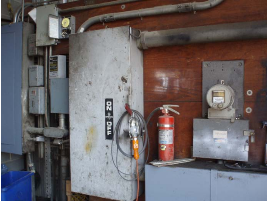
Photograph 13 – Lot 100: Electrical Equipment
