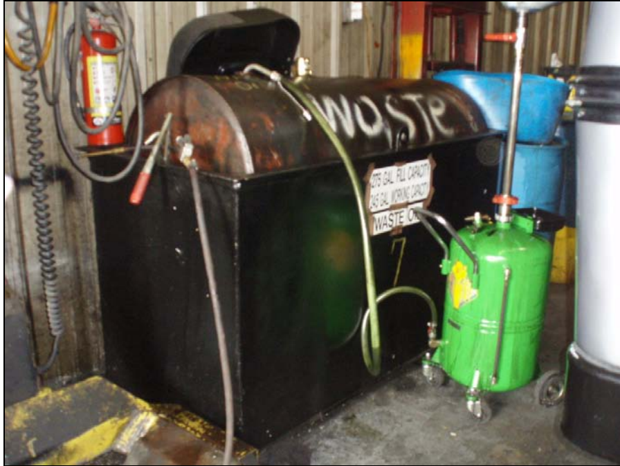
Photograph 5 – Lot 100: 275-Gallon Above Ground Storage Tank
