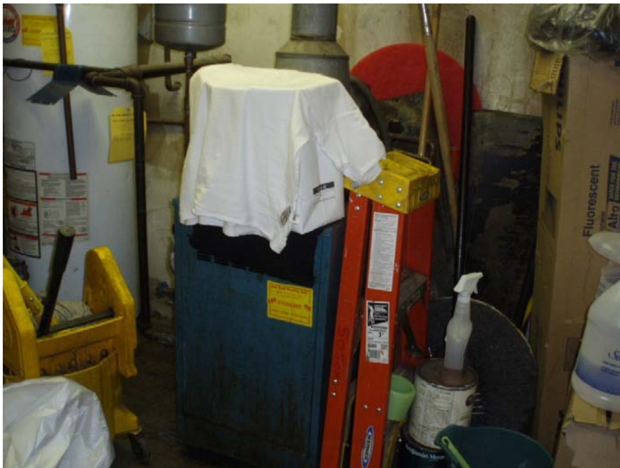
Photograph 14 – Lot 100: Hot Water Heater and Gas Furnace
