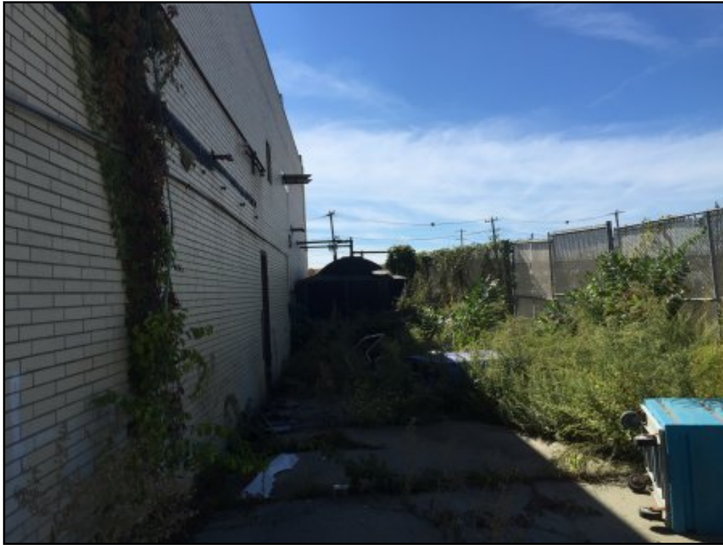
5,000-gallon #2 oil AST, along western wall of eastern-structure
