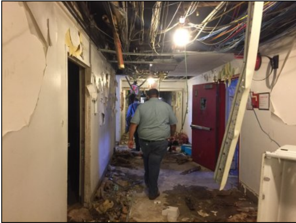
Typical building interior debris
