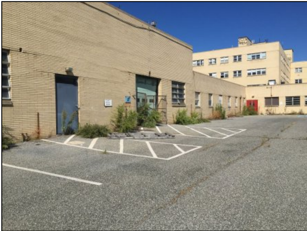
Easterly wall of the furnace room exterior, view facing northwest, note suspected fuel tank fill and vent piping against exterior wall along the left side of the door.
