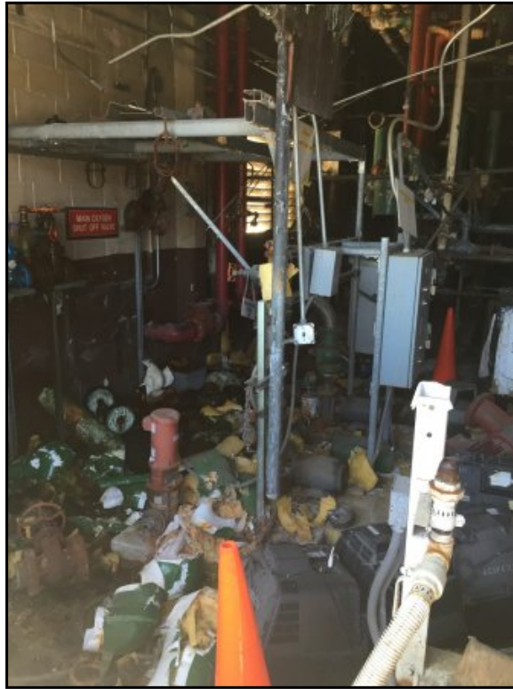
Furnace room interior, note debris and lack of ability to inspect floor area.
