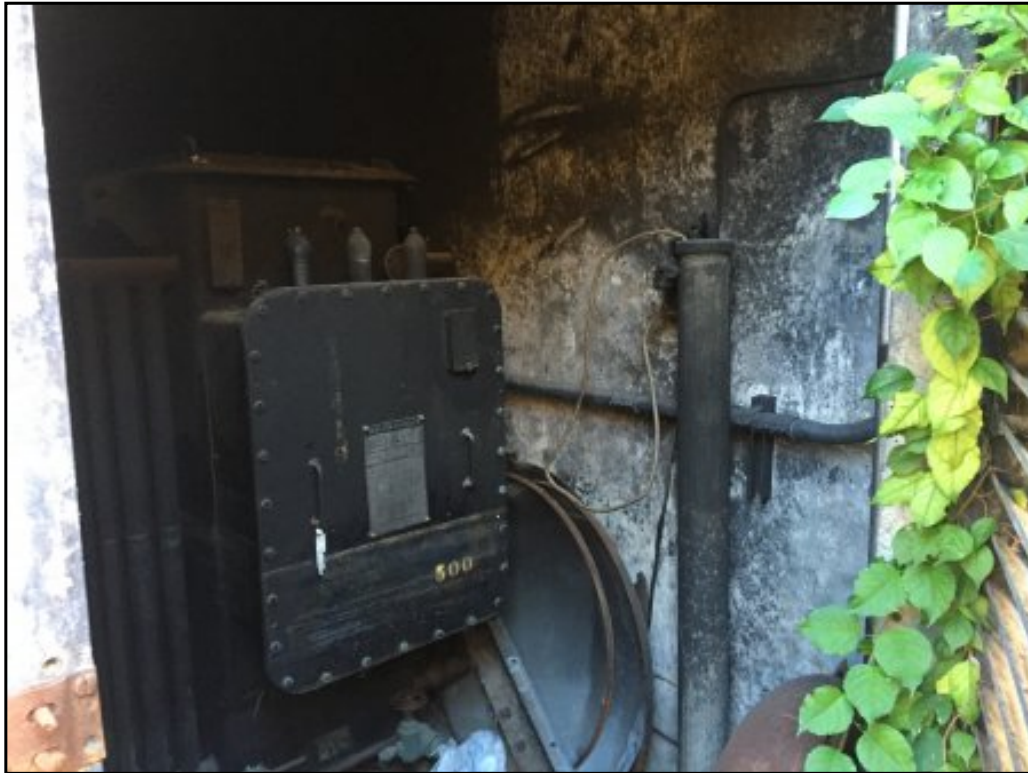
Transformers located along westerly side of eastern structure.
