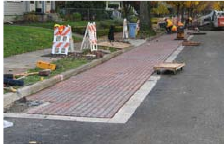
The Portland Bureau of Environmental Services is experimenting with pervious pavers and porous asphalt in residential neighborhoods. In this image, the pervious pavers serve a dual purpose, clearly marking the parking lane as well as reducing rain run-off and flooding. Image used with permission of City of Portland Bureau of Environmental Services.
