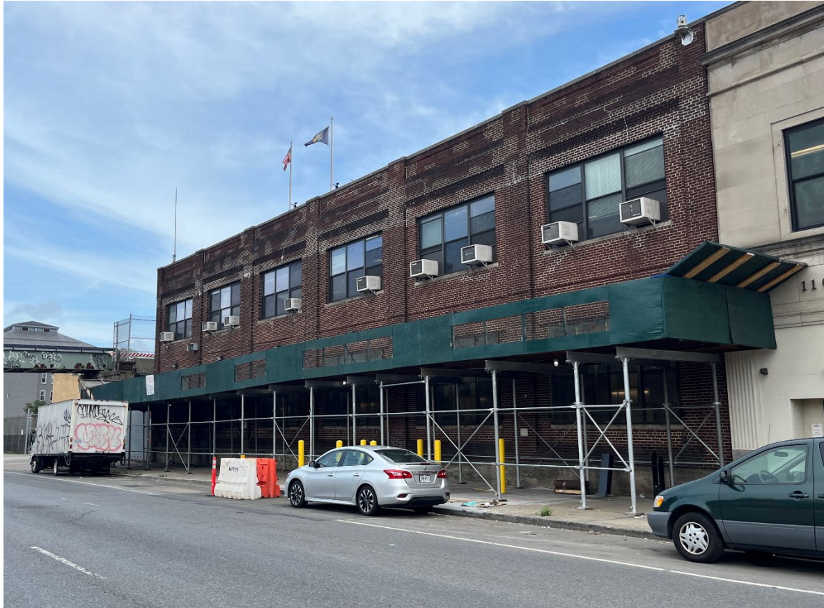
View of the MTA Cable repair and storage buildings, looking south from Atlantic Avenue
