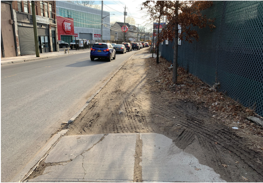
FIGURE 33: Missing sidewalk along Richmond Terrace.
