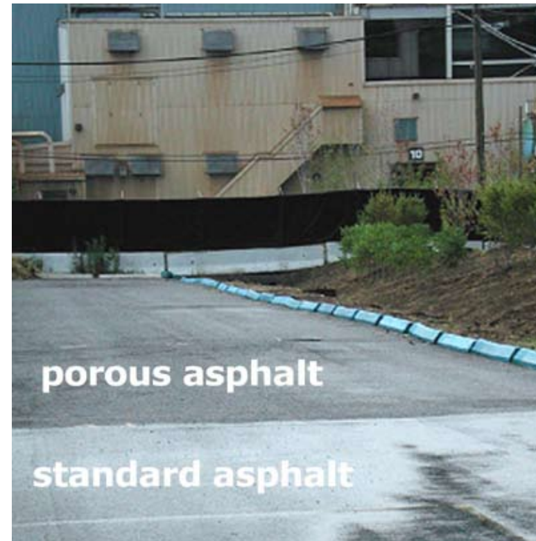
The use of porous asphalt can dramatically reduce the amount of water that remains on the road surface after a storm. This image taken shortly after an intense rainstorm shows essentially dry porous asphalt at the top and water sitting on conventional asphalt at the bottom. Image used with permission of Cahill Associates.
