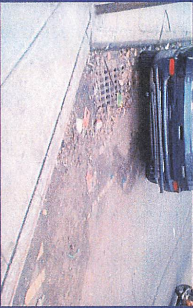
Clogged storm drain 27 th Street
