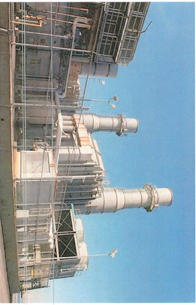
A 'peaker' plant – among the dirtiest forms of energy production in NYC.
