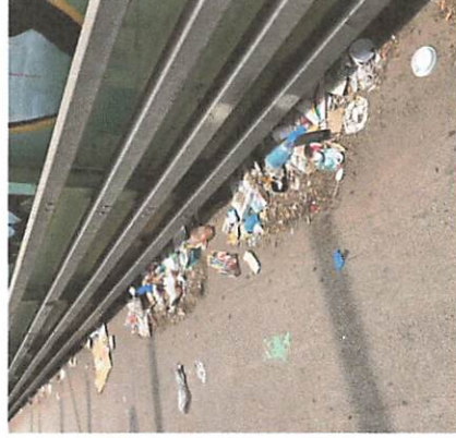
Littering on Queens Boulevard Bridge (East Expansion)
