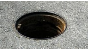
Missing Street Hardware
