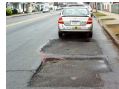
Failed Utility Cut
