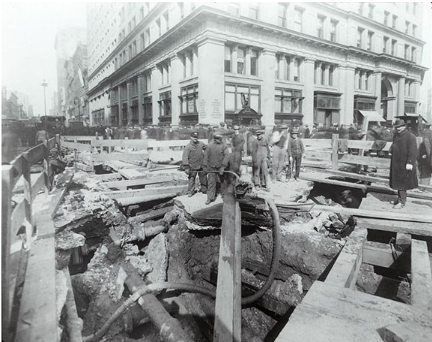
March 1914 photo of a water-main break at 23rd Street & Fifth Avenue.
