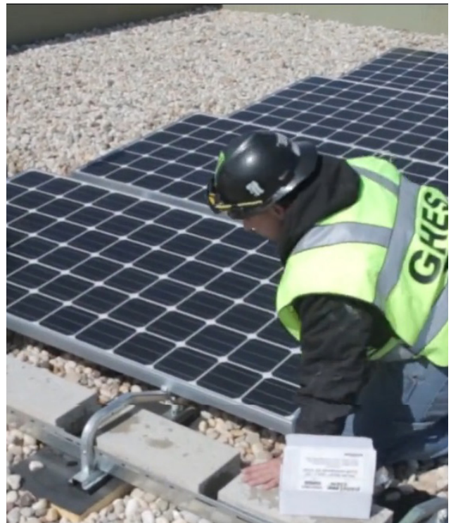
Solar installation in NYC
