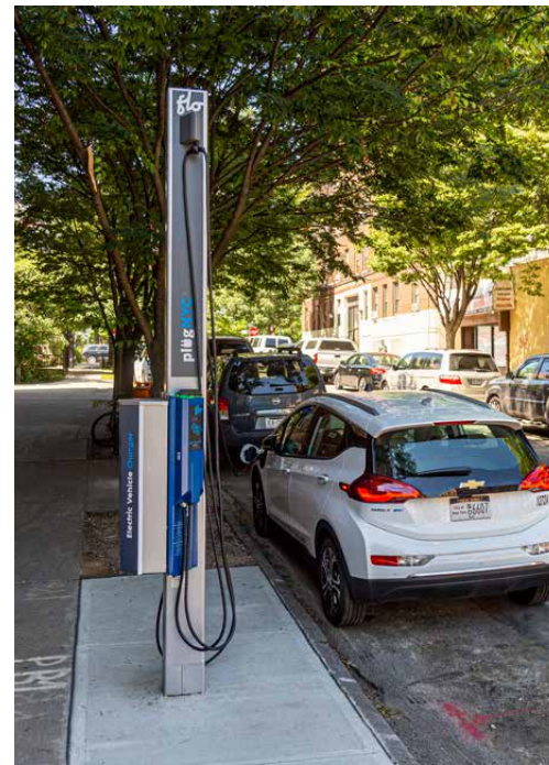
Figure 4.10 Curbside EV Charger
