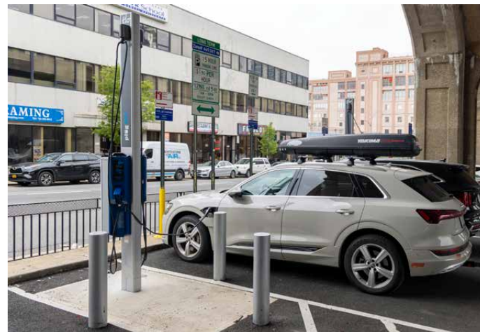
Figure 4.43 Municipal EV Charging Infrastructure
