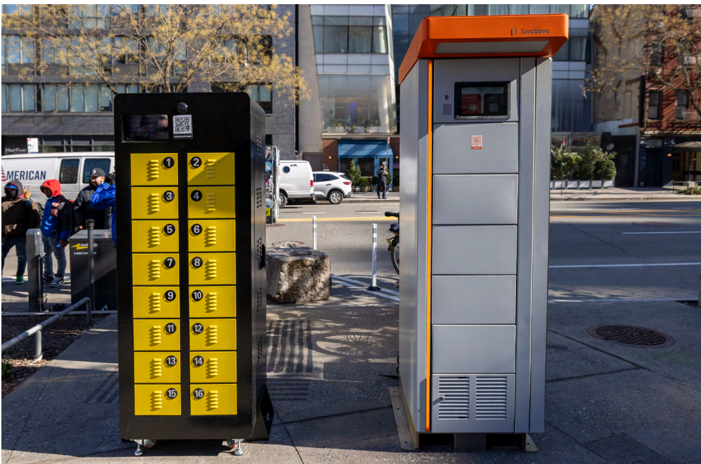
Battery swapping cabinets at Cooper Square as a part of DOT's 2024 E-Bike Charging Pilot Program.
