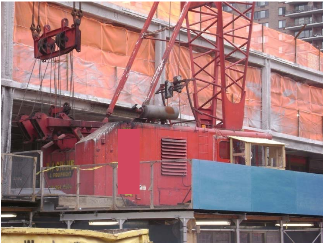
Figure C.6.1: Example of Older Equipment (Site 48)
