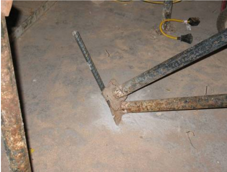
Figure B.6.11: Improper Lateral Bracing Installation, Not in Conformance with Design. Lateral Braces are not Secured to Slab, Unable to Resist Load Reversals
