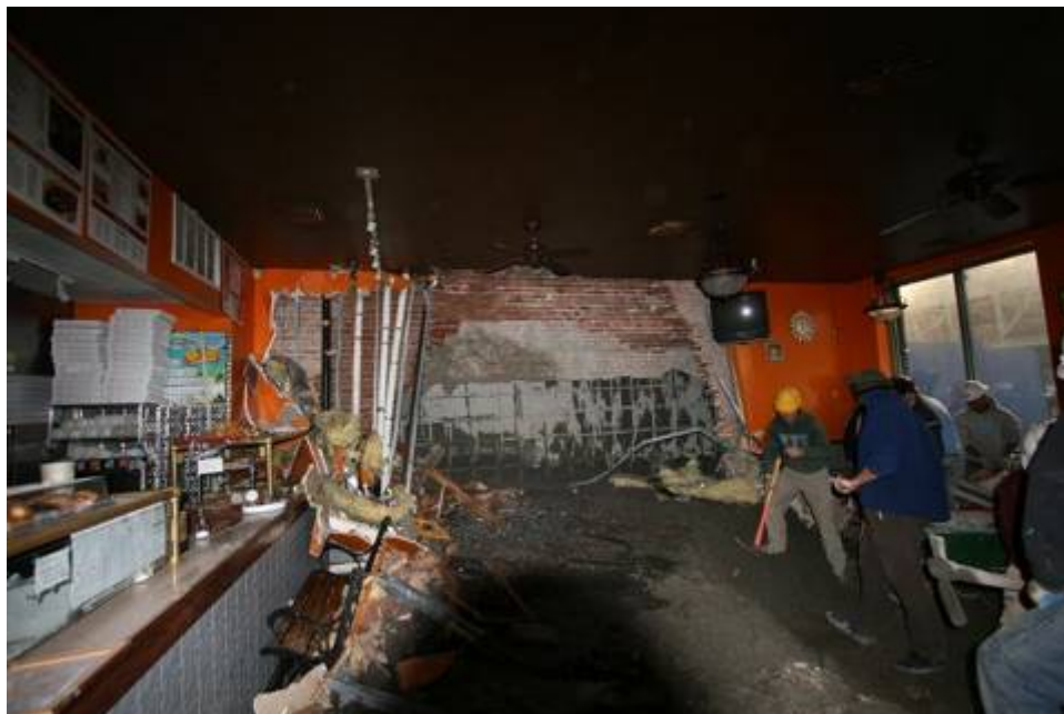
Figure B.6.6: Wall Failure Attributed to Concrete Pressures Imparted by Adjacent Construction
