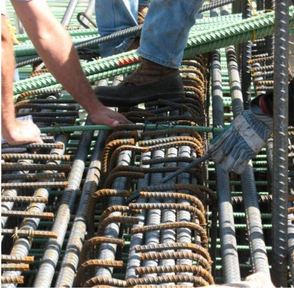
Figure B.10.3: Constructability Issues at Transfer Beam top bars
