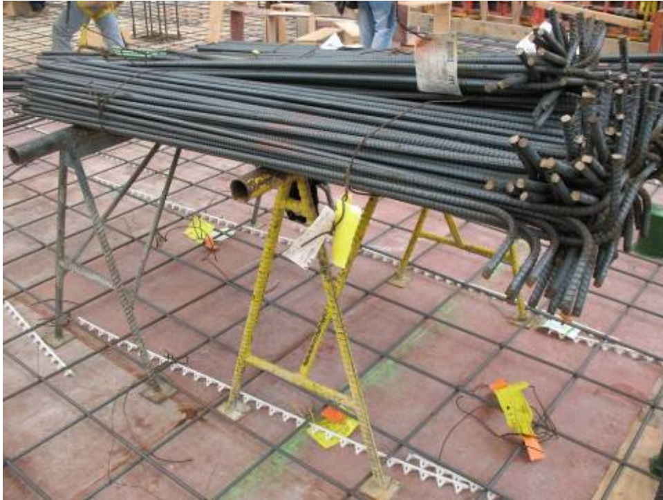
Figure B.6.7: Construction Loads can be Significant 7 . Verification of Proper Formwork Assembly is Critical
