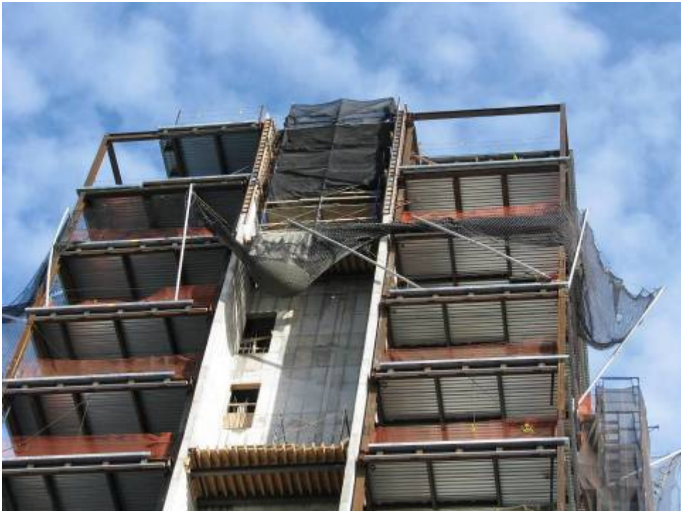
Figure B.6.14: Spilled Concrete after Form Blow-out Restrained by Horizontal Netting (Center)
