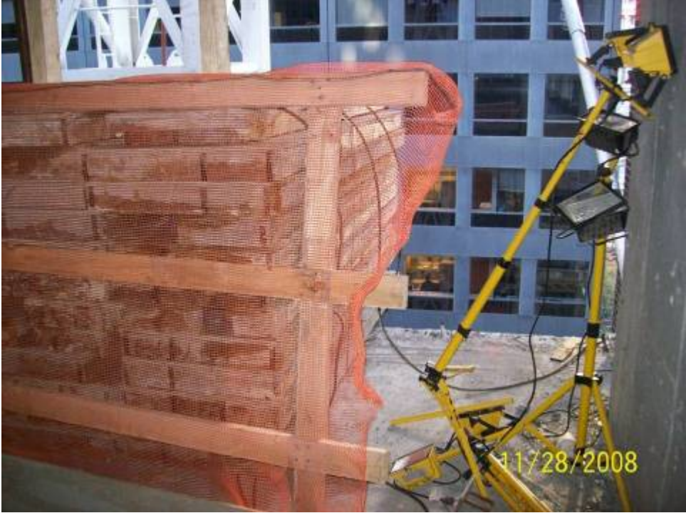
Figure B.7.5: Localized Discontinuous Guardrail Condition at Material Storage Location. Lack of Specificity Regarding Allowable Gap Distances Forces Inspector to Make a Potentially Inconsistent Judgment Call
