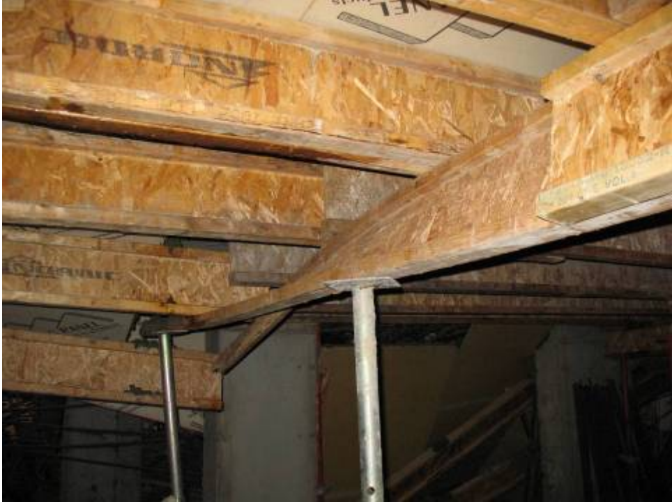
Figure B.6.9: Stacked Engineered Lumber Formwork Failure in Queens Attributed to a Lack of Lateral Bracing.
