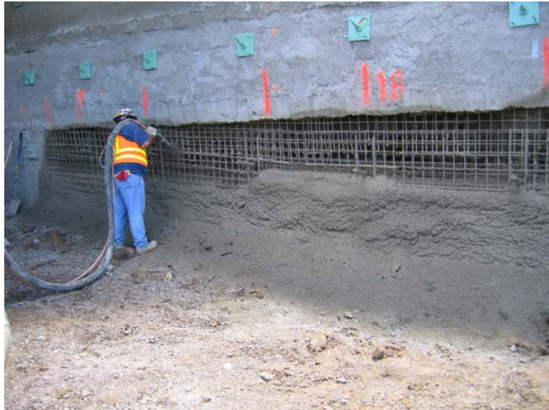
Figure D.16.6: Application of shotcrete over wire mesh for a soil nail wall (Hayward Baker, Inc.)
