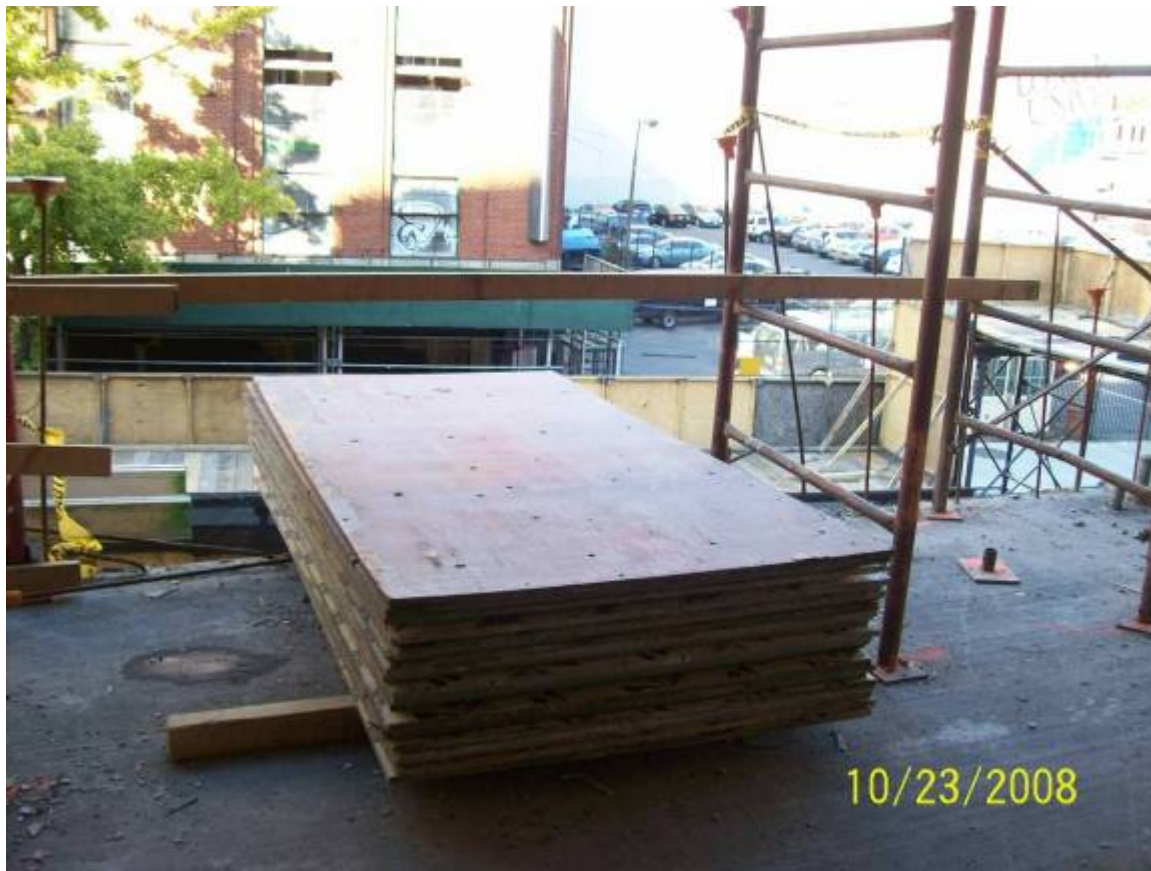
Figure B.7.3: Stacked and Unsecured Material Presents a Wind Borne Debris Hazard When Placed Near Building Edges
