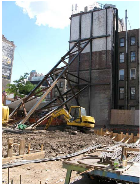
Figure D.7.8: Shoring installed after the 16-inch lean of the existing structure was discovered by the contractor
