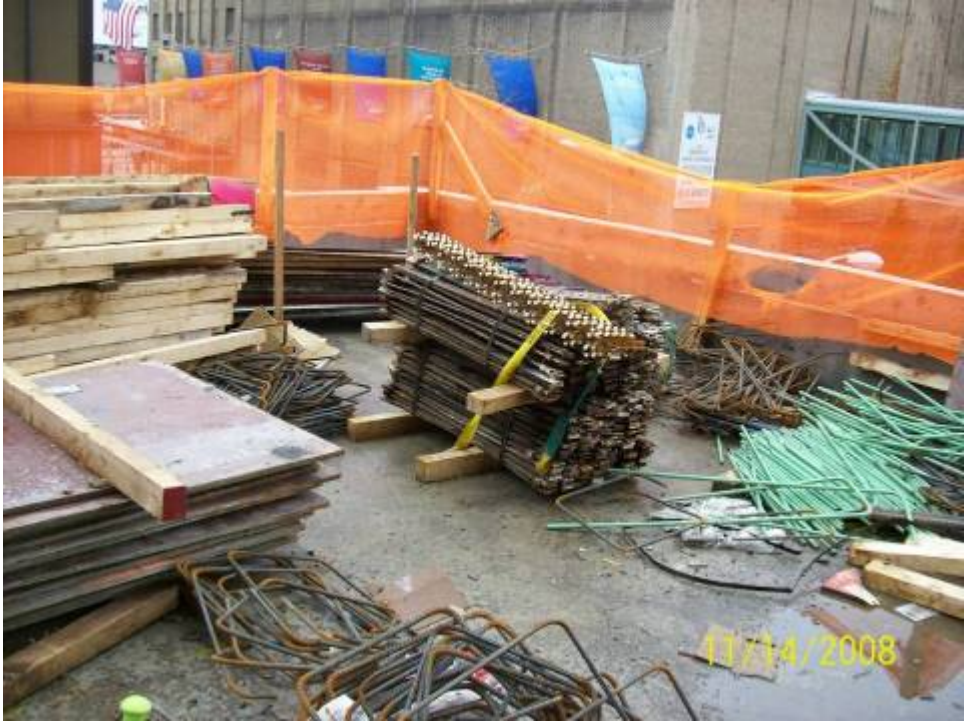
Figure B.7.7: Localized Variation in Guardrail Height. Code Provisions Do Not Address Allowable Height Tolerances (if any). Lack of Specificity Forces Inspector to Make a Potentially Inconsistent Judgment Call
