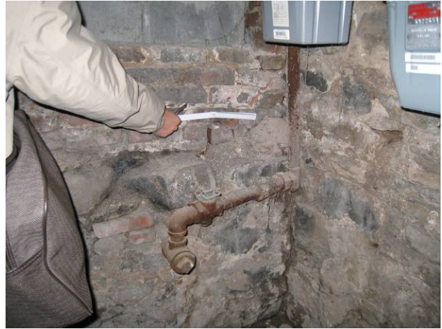
Figure D.10.4: Cracking and lateral displacement of below grade wall during underpinning
