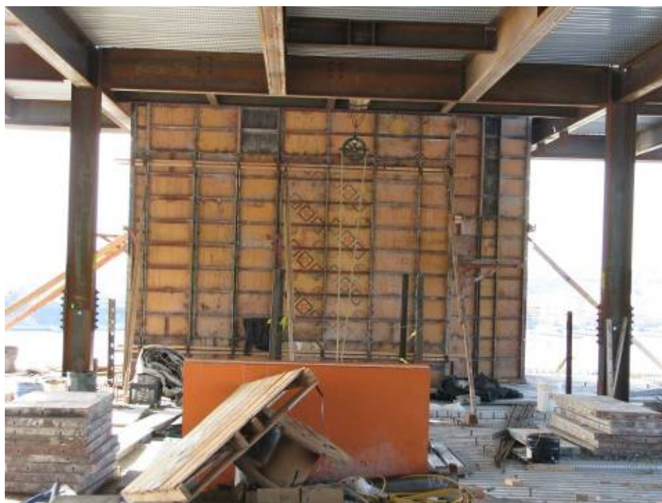
Figure B.6.12: Vertical Formwork Configuration, Missing Walers Specified by Formwork Designer
