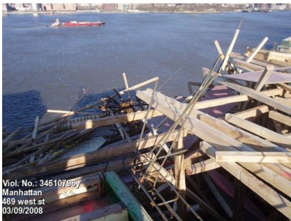
Figure B.6.16: Formwork Failure at Hudson River Exposure
