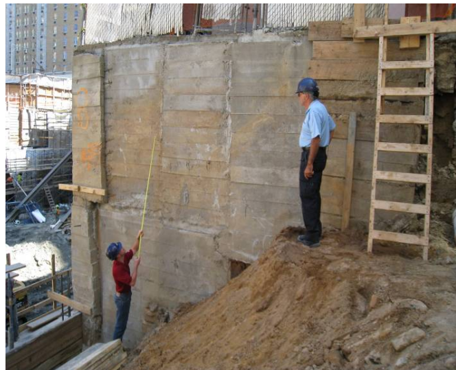
Figure D.8.4: 17-ft Underpinning installed at a rear yard as a retaining wall
