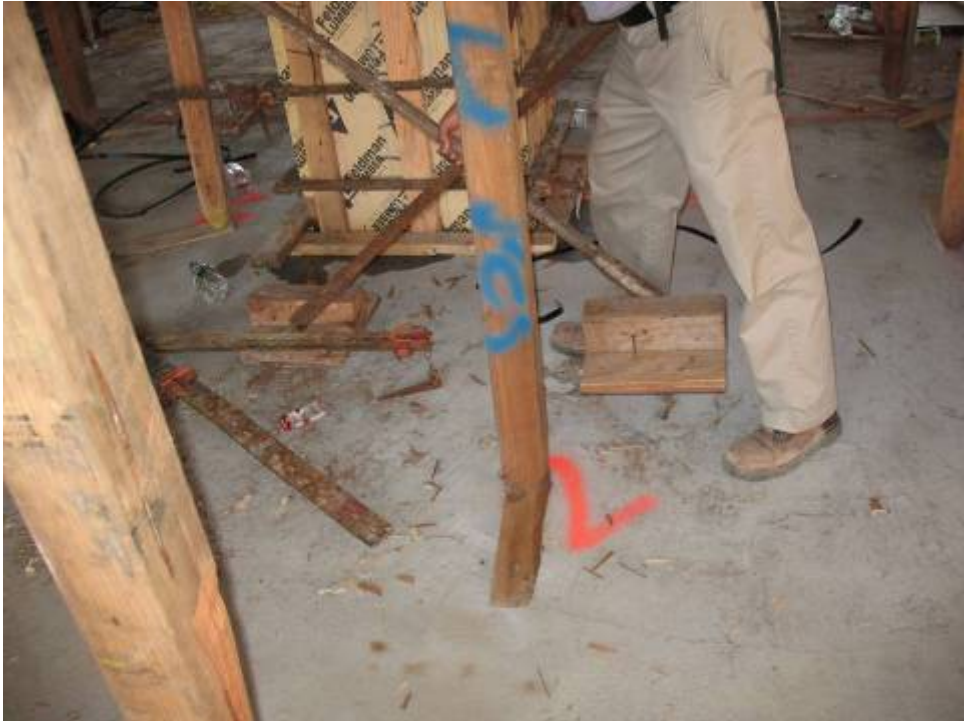
Figure B.6.4: Formwork Construction not in Conformance with Design, Damaged Timber Post
