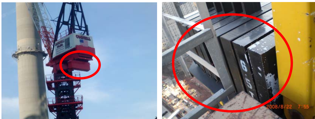
Figure C. 7.14: Crane counter weights
