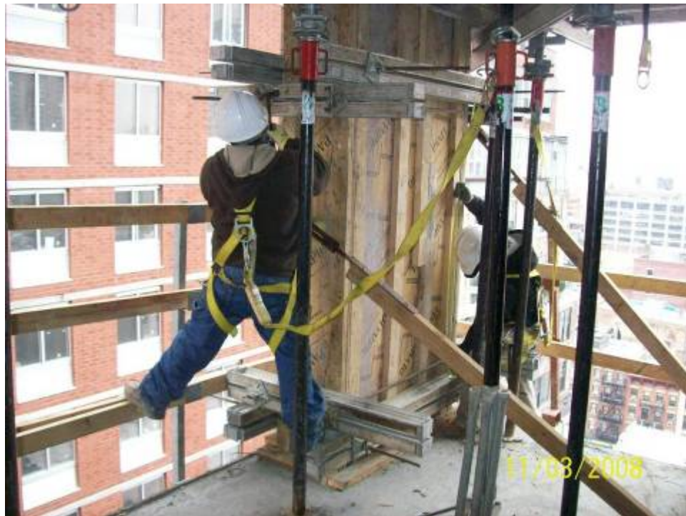
Figure B.8.3: Proper Tie-off. Note Use of Built-in Anchor Points on Engineered Formwork (Prefabricated Steel) Towers
