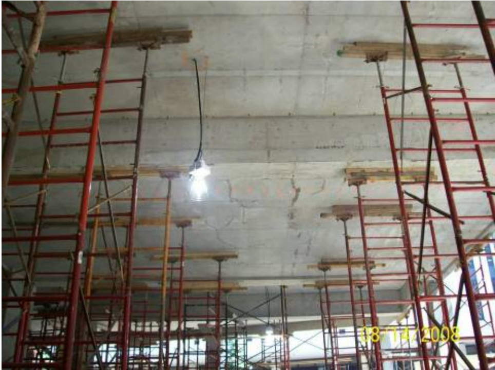
Figure B.6.3: Improved Filler Material Installation (Laid Horizontally) between Steel Shoring Tower and Concrete Soffit
