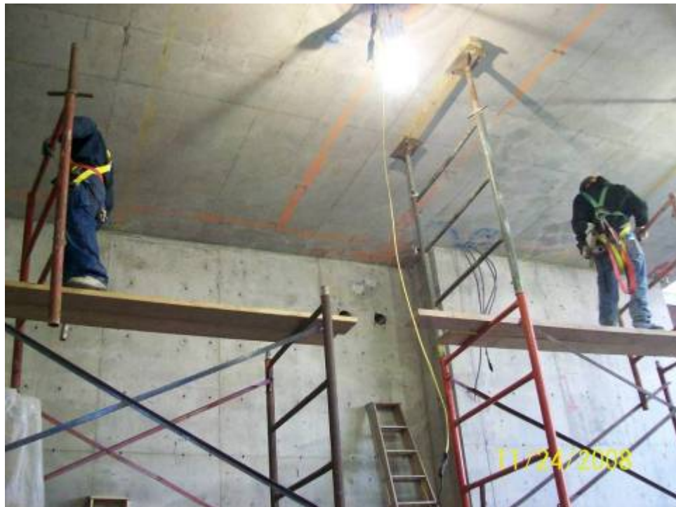
Figure B.8.9: Repeat Failure to Tie-off at Site No. 86, 24-Nov. 2008 (OSHA Violation)
