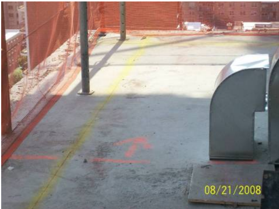
Figure B.7.11: Acceptable Level of Debris Accumulation
