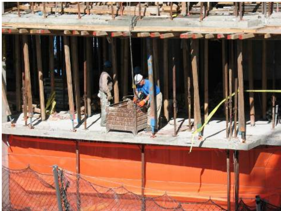
Figure B.7.20: Hoisting of Debris Container (Mini) Requires Rigging Operations at Unprotected Edge. Hoisting Will Also Require Crane “Side-Pulling”. Note Lack of Proper Worker Tie-Off
