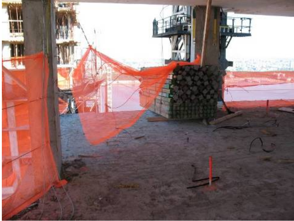
Figure B.7.19: Current Code-Compliant Material Storage Practice (Piled Material is Banded and Braced) and Accompanying Fall Hazard at Unprotected Edge (Left)
