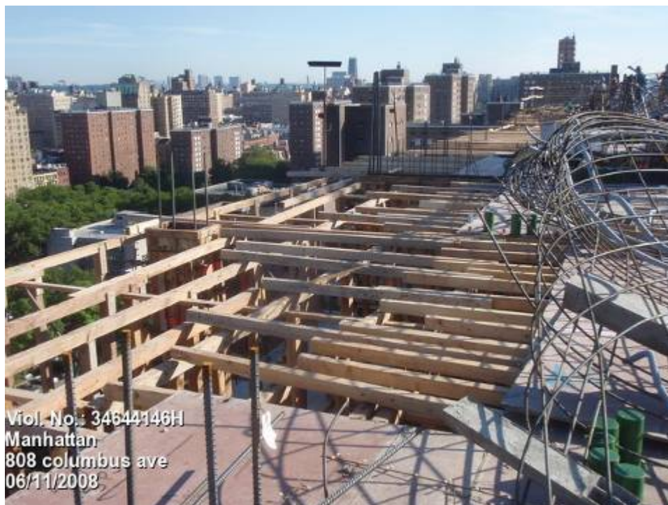
Figure B.6.17: Formwork Failure in Reported 30-40 mph Winds
