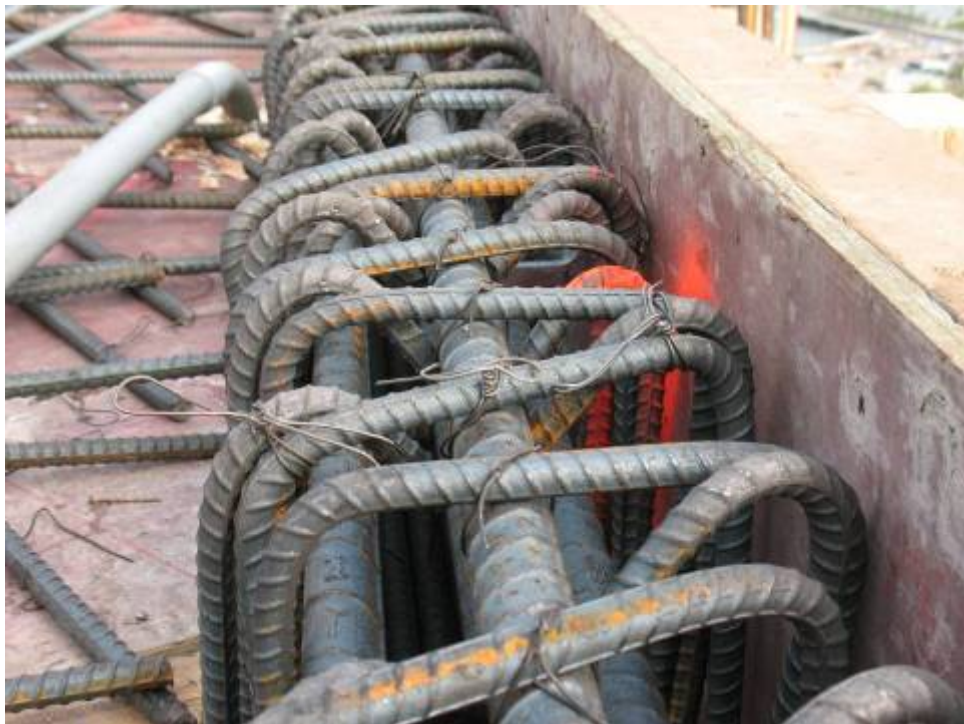
Figure B.9.4: Typical Critical Quality Defect: Bar Congestion and Improper Shear Stirrup Engagement. Conditions Subsequently Remedied to the Satisfaction of the Engineer of Record
