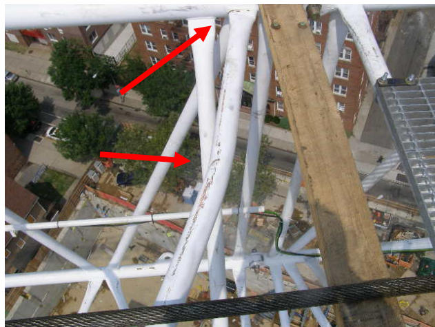
Figure C.10.4: From DOB incident / accident files
