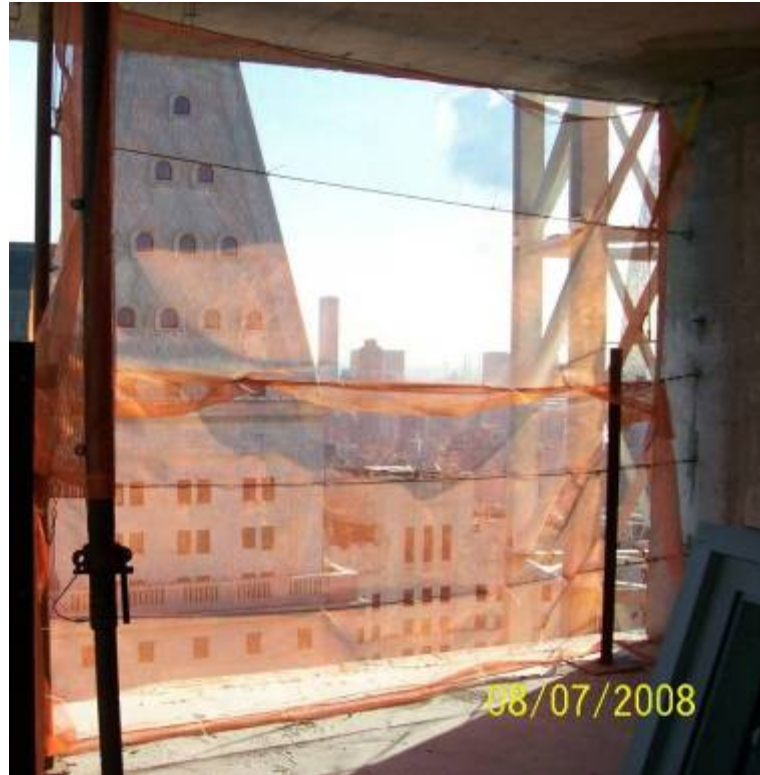
Figure B.7.14: Full-height Vertical Netting Provides Additional Barrier to Flying Debris
