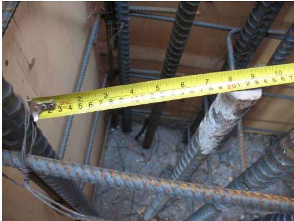
Figure B.9.1: Typical Critical Quality Defect: Column Splices Noncompliant with ACI. Conditions Subsequently Remedied to the Satisfaction of the Engineer of Record
