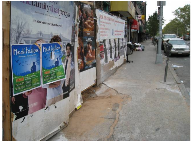
Figure D.10.6: Localized soil loss and structural collapse of unsupported sidewalk
