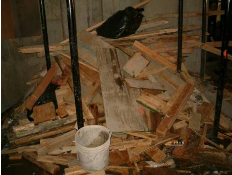
Figure B.7.10: Unacceptable Level of Debris Accumulation Presenting a Major Impediment to Egress. Enforcement Level: Stop Work Order
