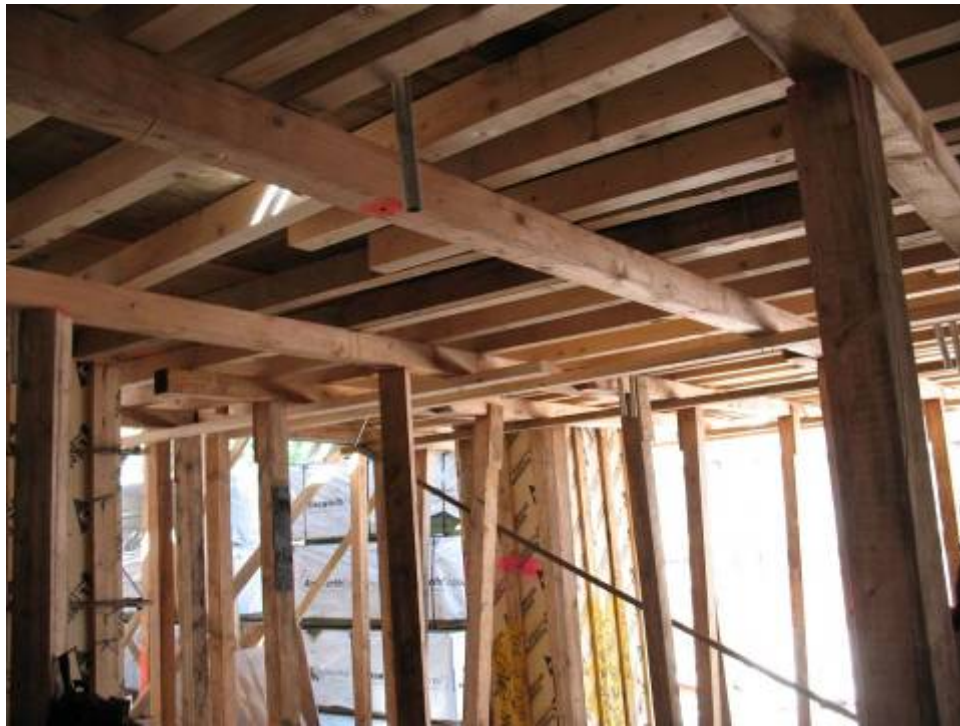
Figure B.6.5: Insufficient Post Spacing, Missing Posts at Stringer Element (Top Center)
