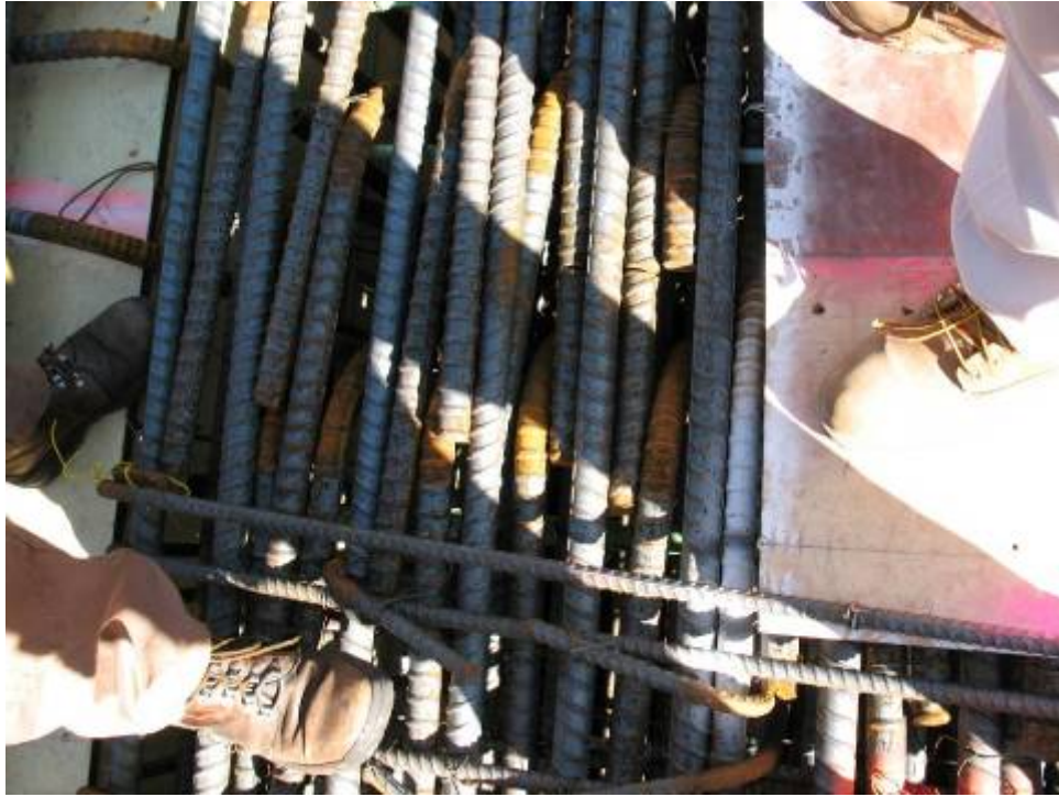
Figure B.9.10: Severe Bar Congestion 29 . Conditions Brought to the Attention of the Engineer of Record
