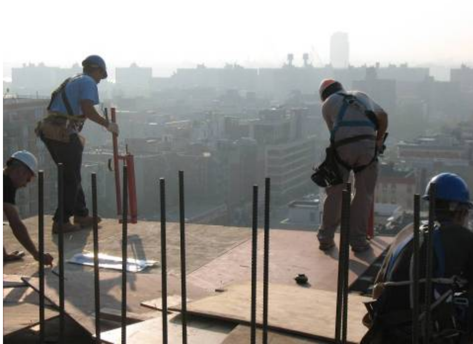
Figure B.8.1: Failure to Tie-off During Decking Operations. Retractable Lanyards Could Have Been Utilized, Anchoring to Formwork Subassembly
