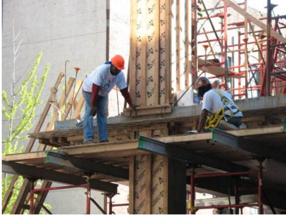
Figure B.8.8: Repeat Failure to Tie-off at Site No. 86, 10-Sept. 2008 (OSHA Violation)
