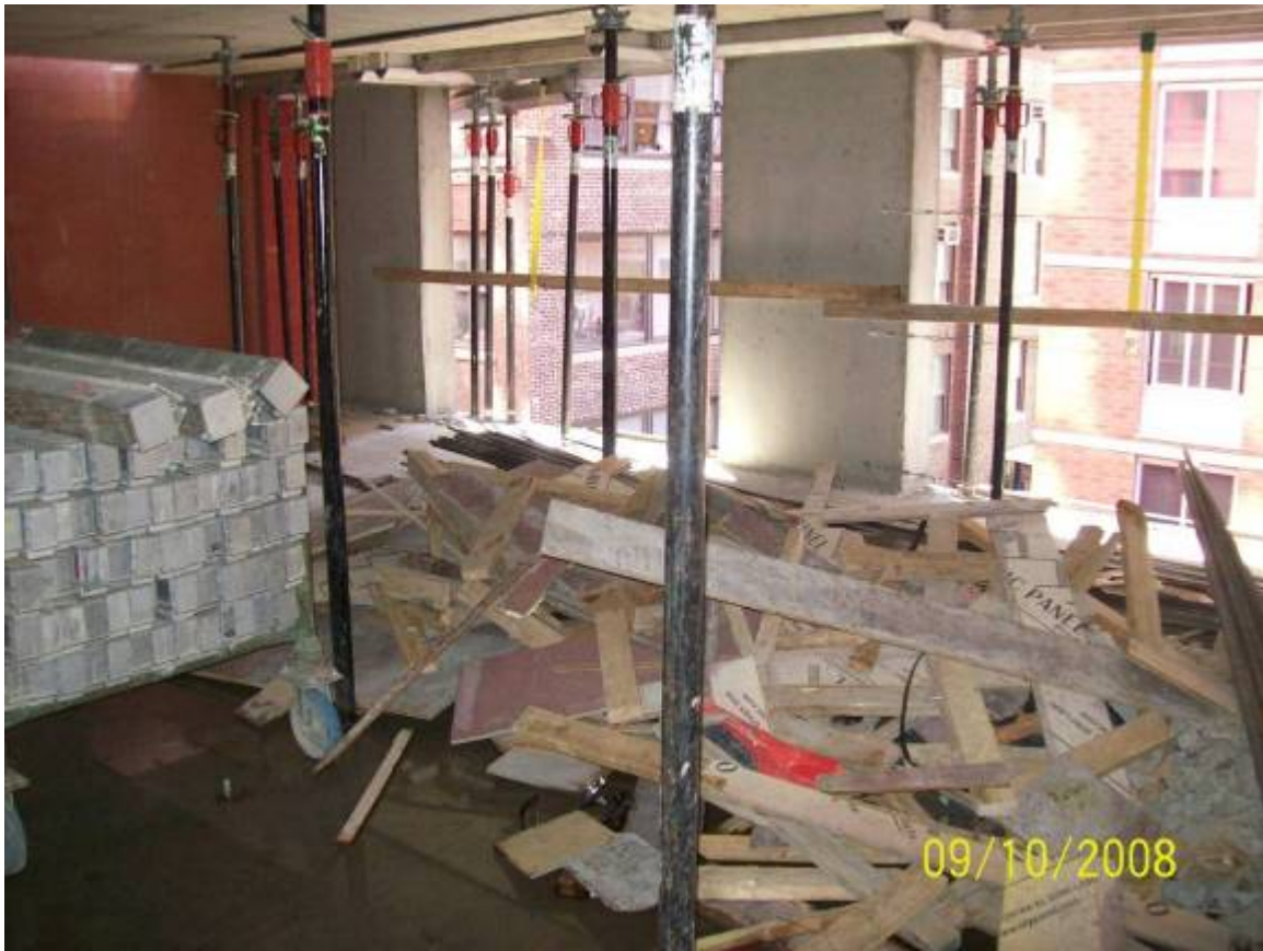
Figure B.7.1: Debris Accumulation Presenting a Public and Worker safety Hazard. Note Unprotected and Unsecured Building Edge (Background).
