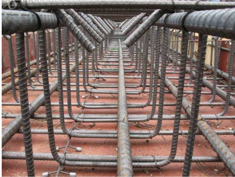
Figure B.9.11: Second Floor Transfer Girder with Improperly Developed Shear Reinforcing. Site No. 47
