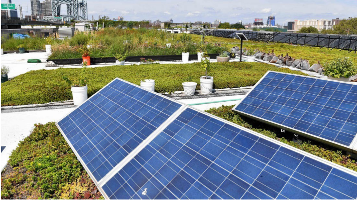
Five Borough Administrative Building 15 Bronx Shore Rd, New York, NY 10035 Completed July 2015 87.80 kW
