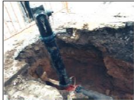
Installation of a new fire hydrant at Quintard Street and Reid Avenue.
