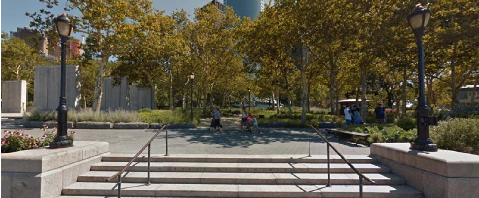
RIVERSIDE LUMINAIRE ON B-POLE WITH RECEPTACLE LOCATED ON EITHER SIDE OF PARK STEPS
