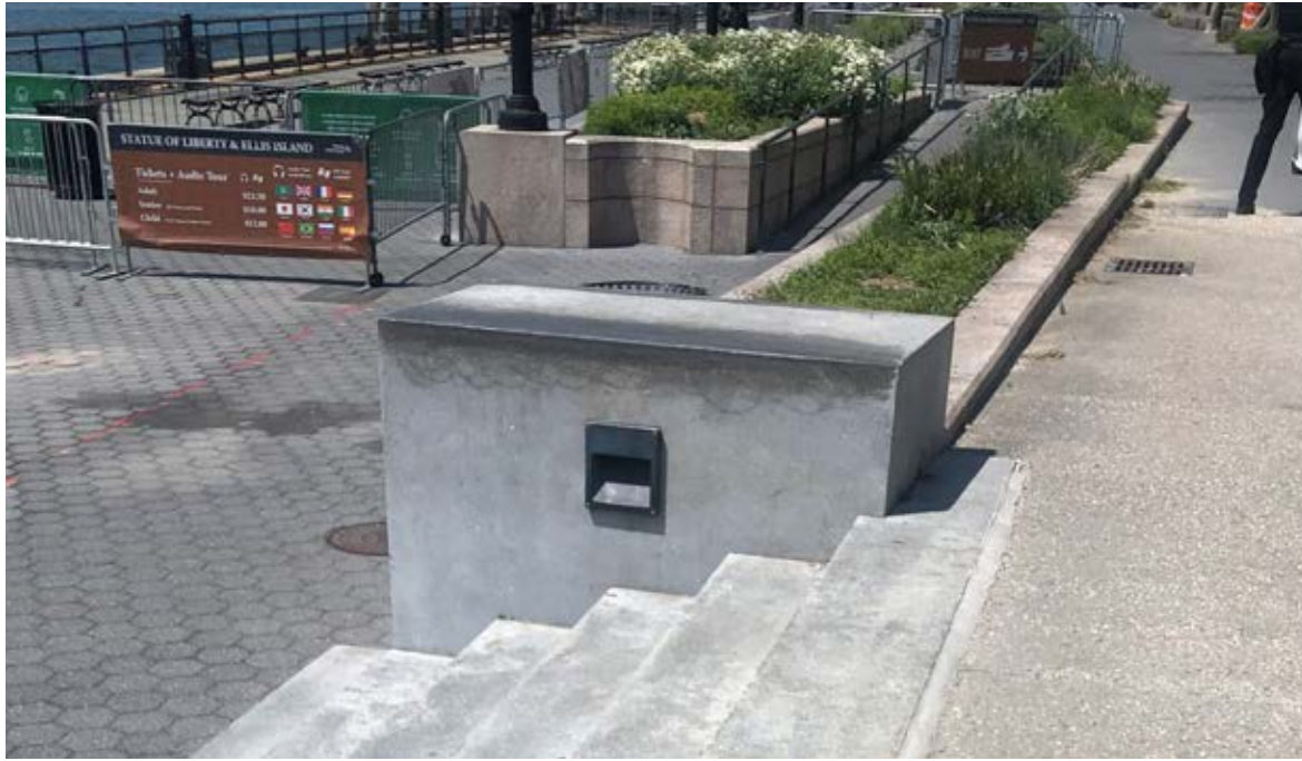
RECESSED LIGHT FIXTURES WITHIN EAST COAST MEMORIAL'S CHEEK WALLS LOCATED ON EITHER SIDE OF EAST COAST MEMORIAL STEPS
