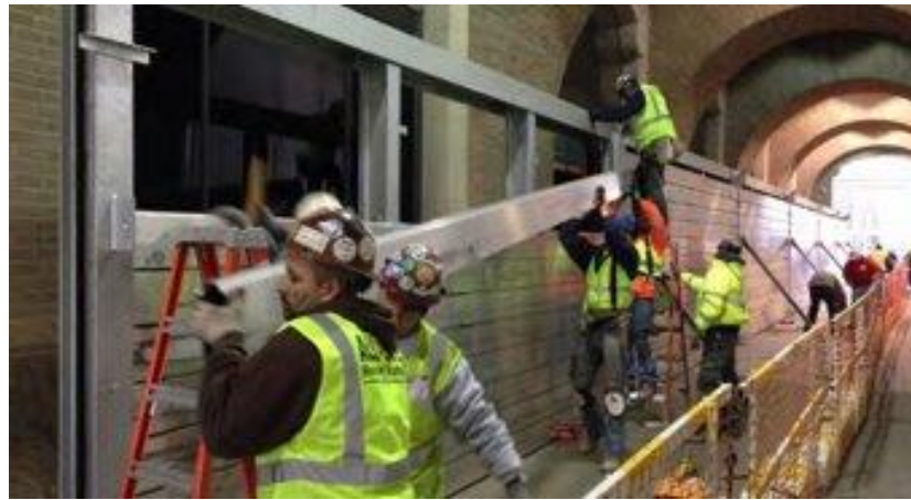
Stop Log / Plank System
